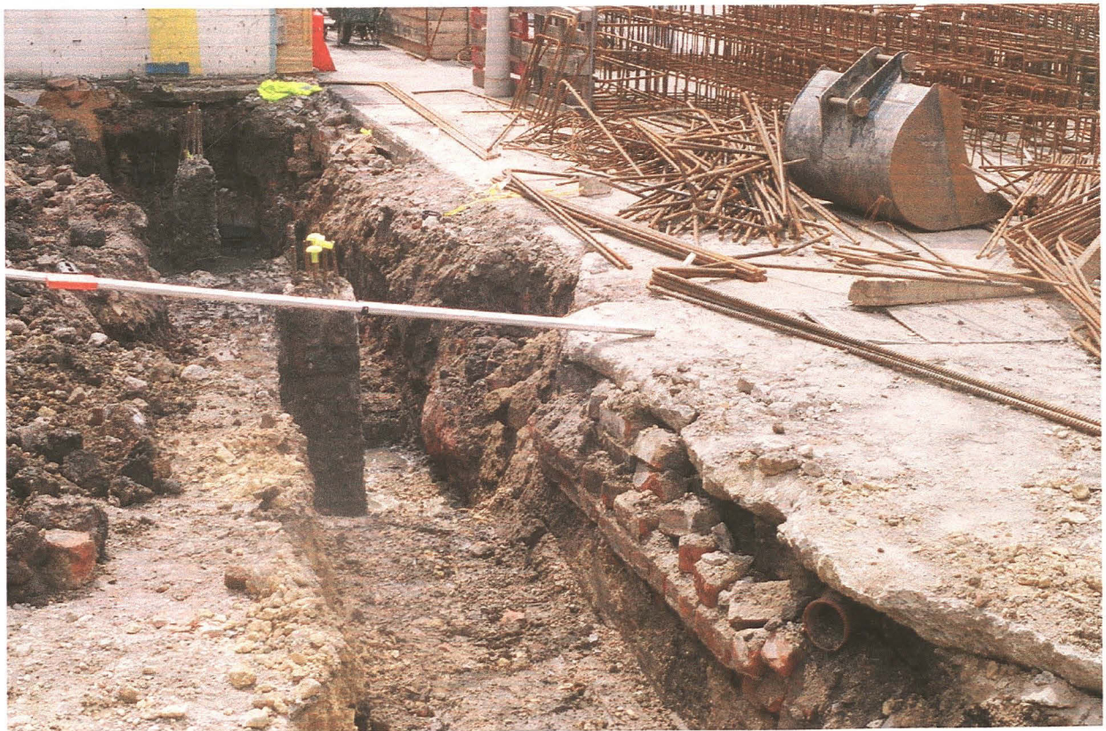
Pl. 8 Looking south west along the foundation trench immediately east of the boiler house, showing concrete piles and 19th century foundations
