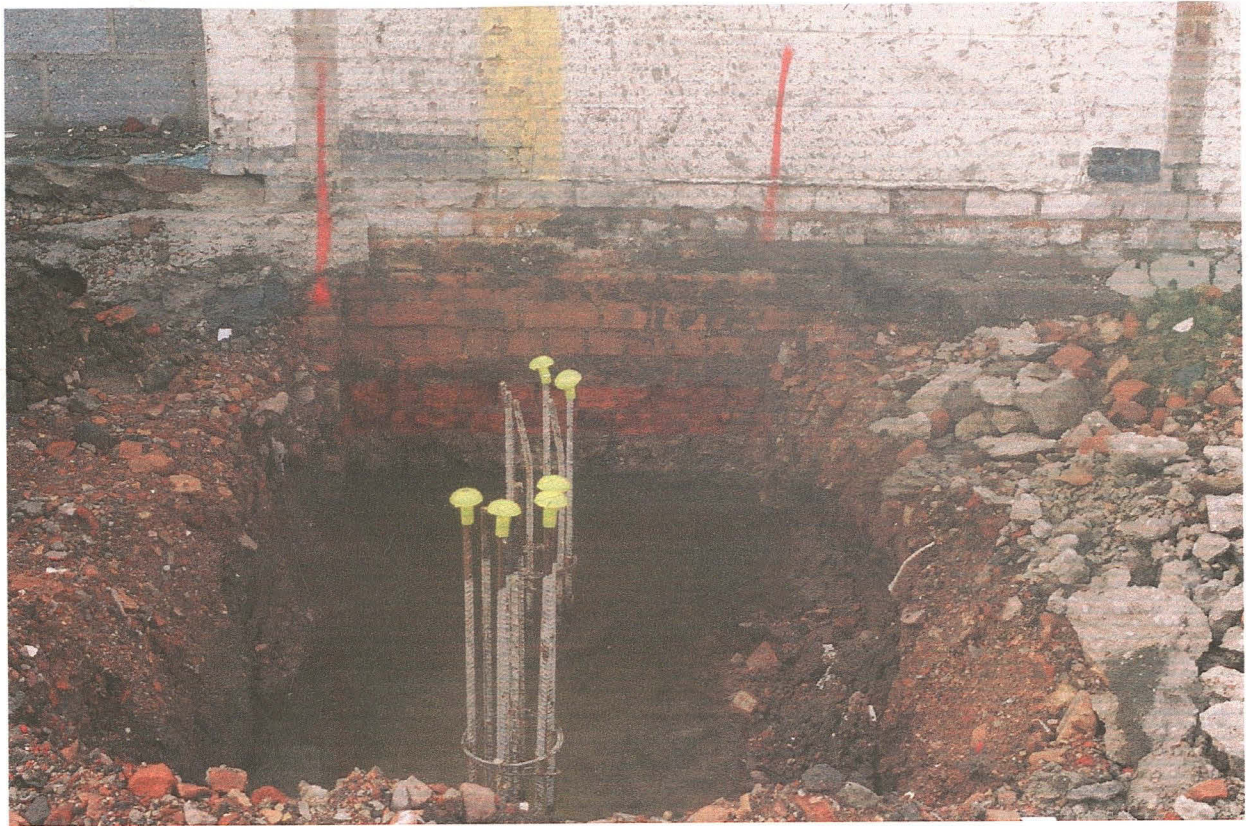
Pl. 7 Looking south at the north facing wall of the existing laundry building showing pile caps, disturbed ground make-up and the relatively high water table
