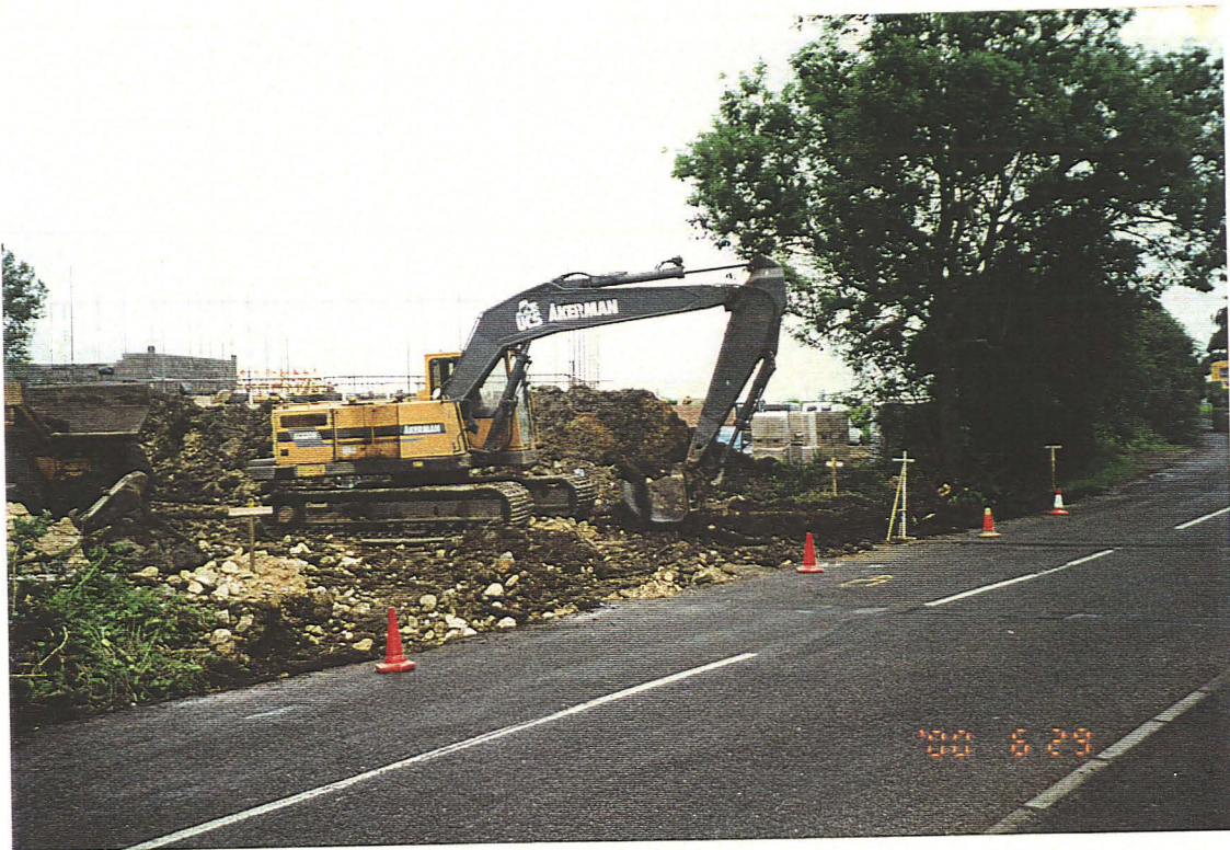
P9. General view of Phase I access road stripping, looking north-east from Scothern Lane
