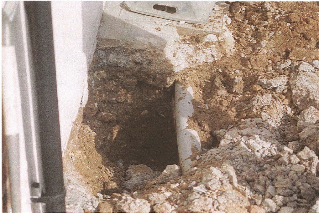
Pl. 22 Limestone rubble extending below the front wall of 'Persian Oasis' at 21. Roman material was found in the mixed deposit below (looking north).
