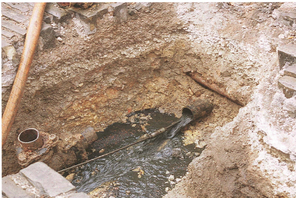
Pl. 16 The existing pipe at 20, being scraped and flushed, was laid immediately above limestone. Beyond the trench backfill are layers of stone chips and rubble, which may represent Roman or medieval metalling of Steep Hill (looking west).
