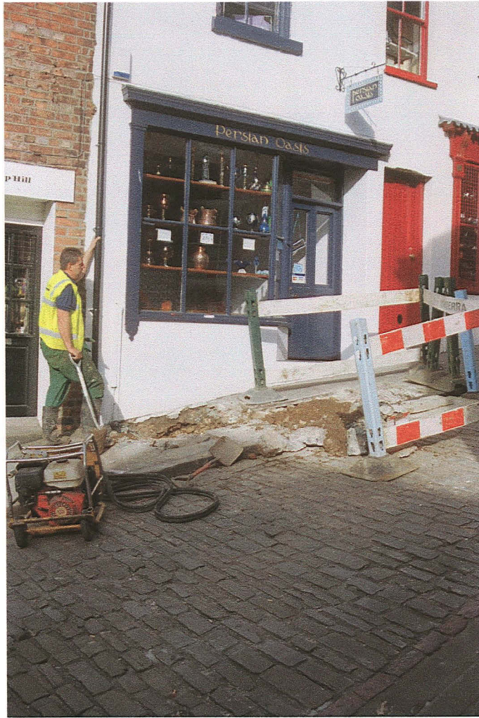
Pl. 20 Location of trench 21 in the western pavement of Steep Hill (looking NW).
