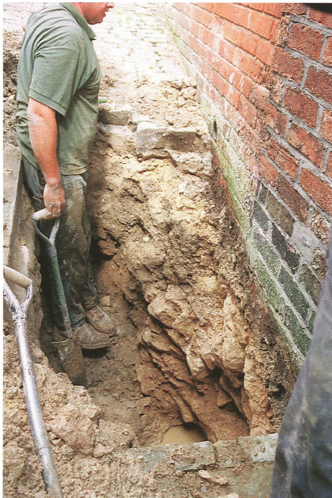
Pl. 23 Setts covering stone rubble core of the Roman wall in Motherby Hill 25 (looking NE).
