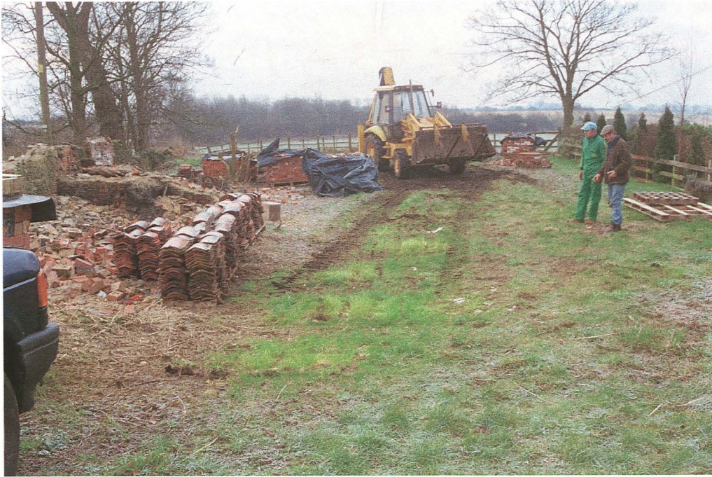
Pl. 1 The building plot (looking south). Part of the southern wall of the Old Blacksmith's Shop remains, abutting the eastern boundary wall.
