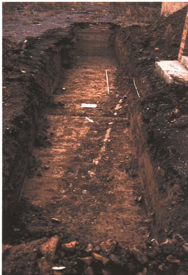
Plate 2: Trench 1, showing drain from the church running diagonally across trench, with the steps at the entrance to the church near top right, looking south-west.
