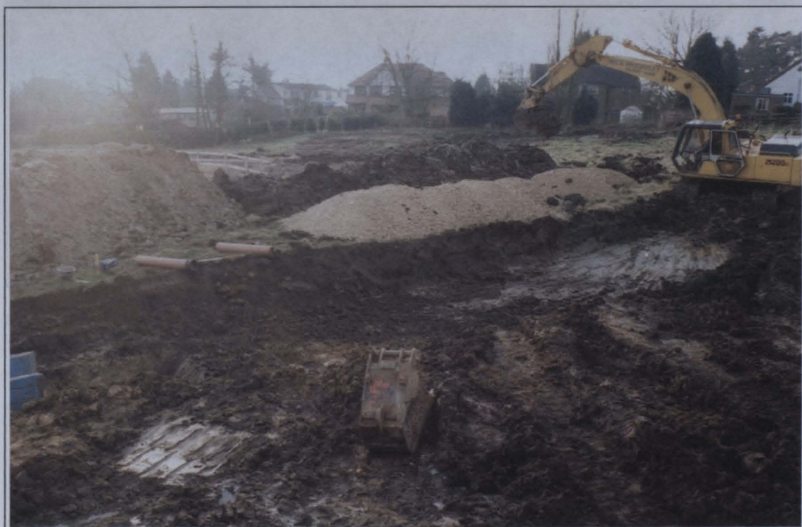
Plate I: General view looking south-west showing the removal of waterlogged soil in the area of Roadway 5A to enable the insertion of surface and foul-water drains.
