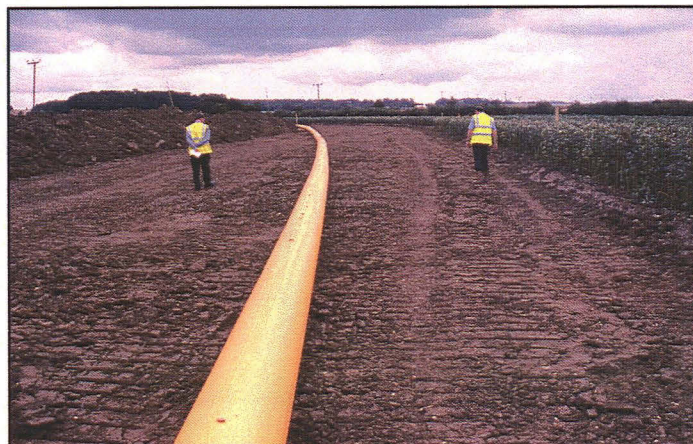
Plate 2: Fieldwalking being carried out on the previously topsoiled easement in Field 4, showing the rutted and weathered condition of the strip.
