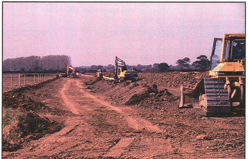
Plate 12: Working shot: trenching, pipe laying and back-filling in Field 14, looking W (pipe joining in background).
