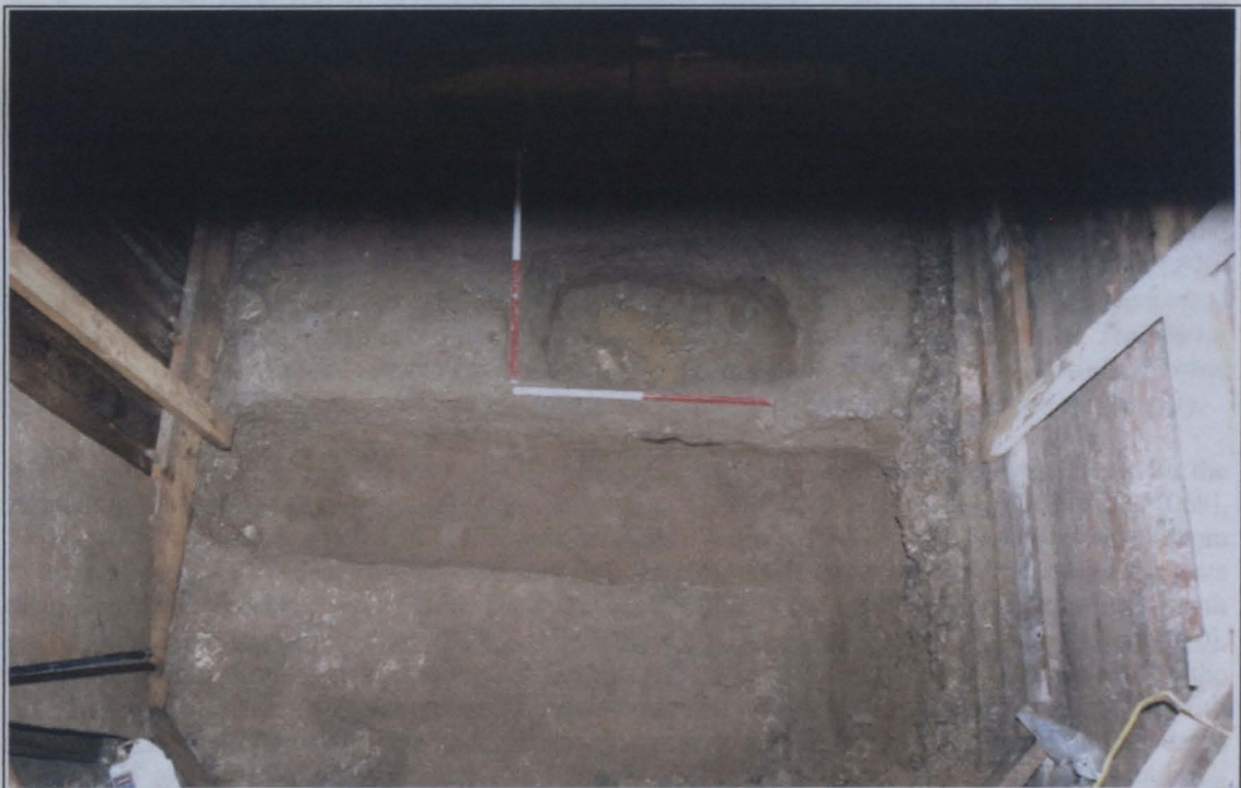
Plate III: Lift pit B looking north, showing east-west construction cut for wall/foundation [039/120] (scales are 1m).
