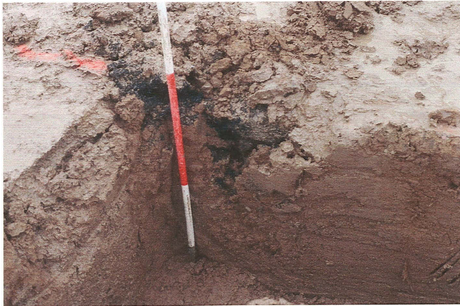
Fig. 4 Area of black asphalt exposed in the south west corner of the building foundation
