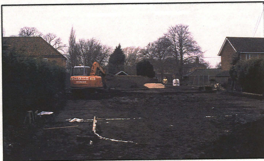
Plate 1 (left): general view of the site during topsoil stripping, looking NW towards Main Street.
