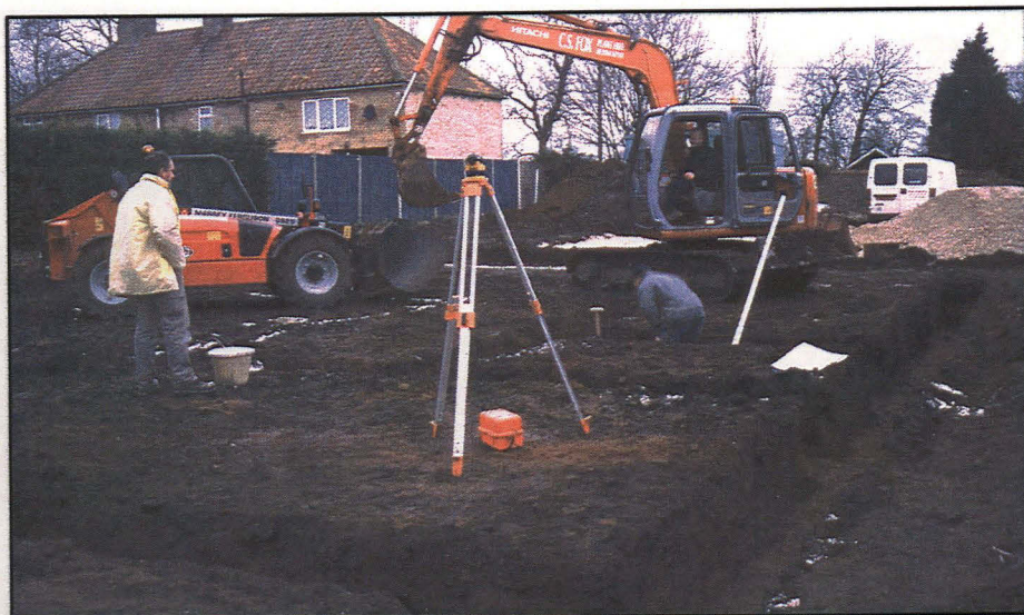
Plate 3 (left): general shot of the site during the excavation of the house foundation trenches, looking SW.
