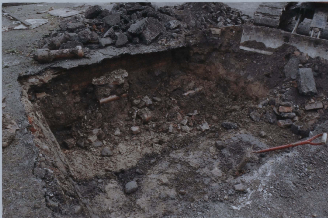
Pl. 6 Trench 2 during machine excavation showing the instability of the ground, looking east
