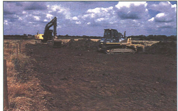
Pl. 12: General view of topsoil stripping in Field 23. The 360° is stripping the easement, which is then bladed flat by the bulldozer and the spoil mounded up. Note the extensive rutting. Looking north
