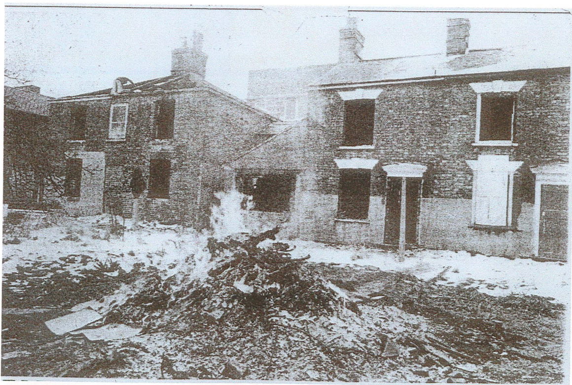
PI. 4 Demolition of properties in Crescent Gardens, 1979 (Spalding Free Press, 27/2/79. Reproduced courtesy of Lincolnshire Free Press).
