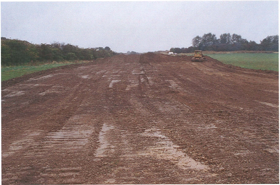
Pl. 1 Bulldozer stripping showing 100 and faint traces of the former stream channel 102 (looking SW).
