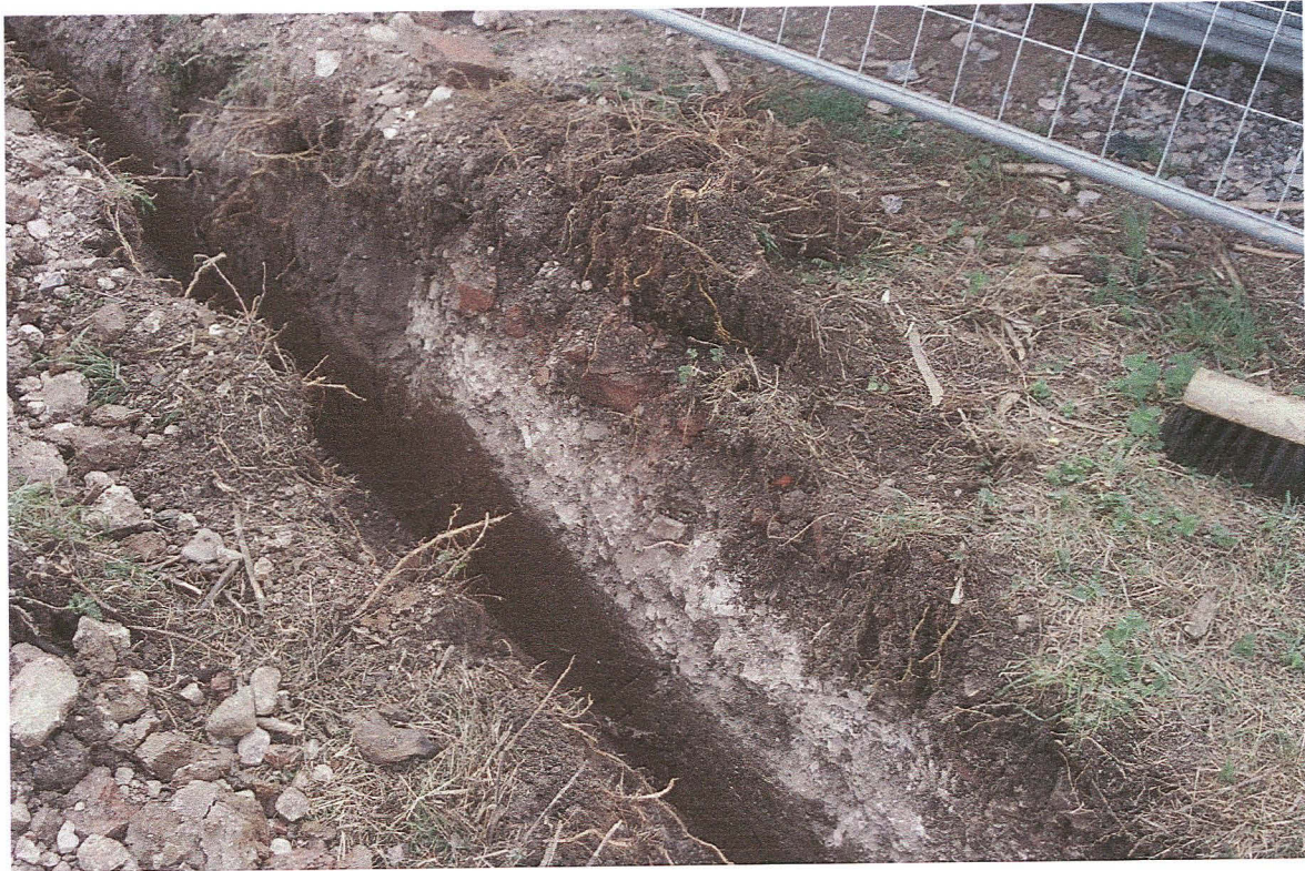
Pl. 3 Brick demolition rubble and track make-up material in trench for electricity cable, Vacuum Pumping Station site, Great Carlton (looking NE).
