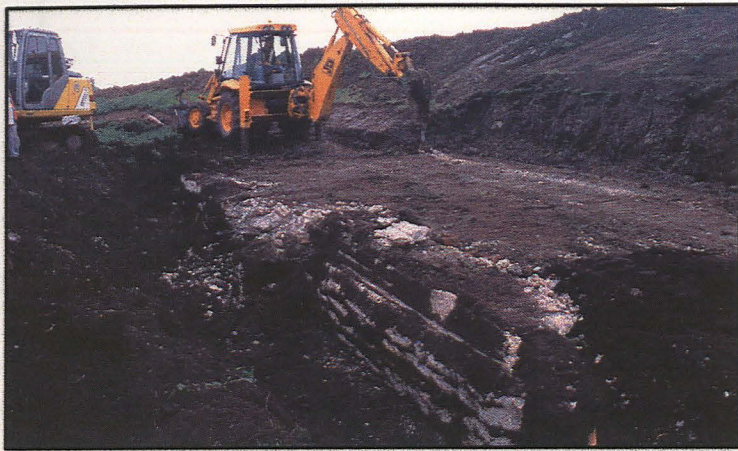
Plate 7: A rockbreaker removing the concrete and brick foundation at ch.41821, looking NW.
