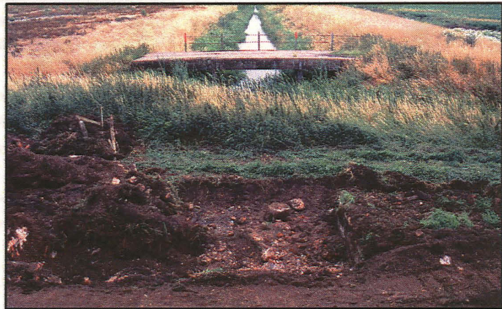
Plate 8: The remains of the pumping station at ch.41850, looking S.
