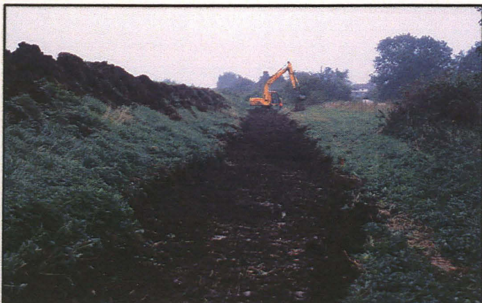
Plate 14 (right): view of the eastern part of section 9, from ch.36650, looking E.
