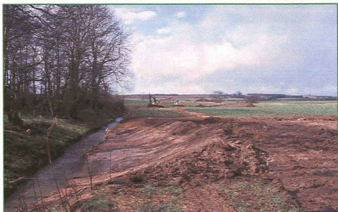
Plate 2 (left): General shot of the development area, showing the completed Area 3 in the foreground, and work in progress on Area 4 in the background, looking W.
