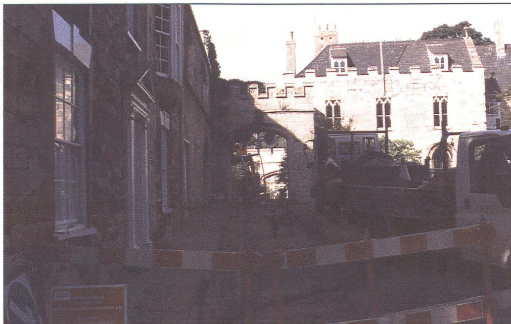
Pl. 1: View along the line of the cable trench, looking west from the east end of the trench.
