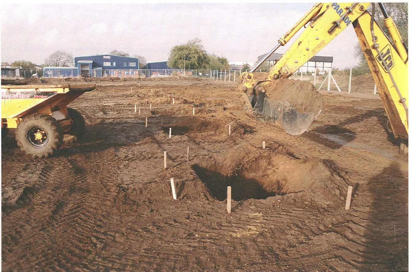
PI.2 Excavation and layout of the eastern alignment of pad foundations, facing north.
