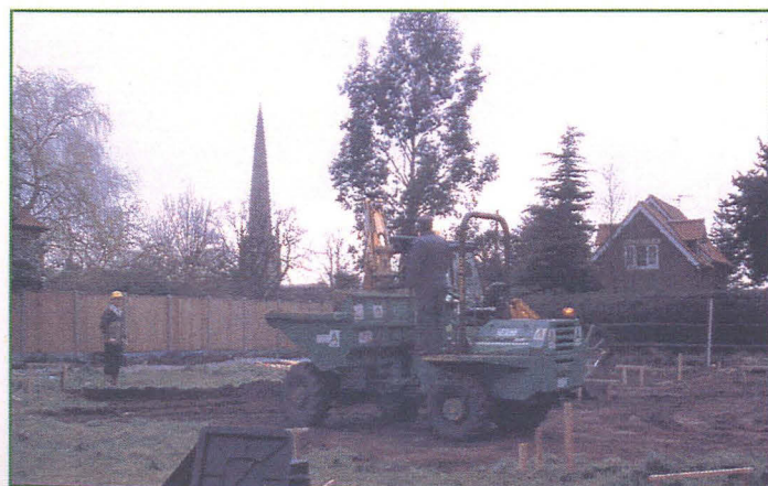
Plate 4 (left): Working shot: topsoil stripping in the house footprint, looking NNW towards the church.
