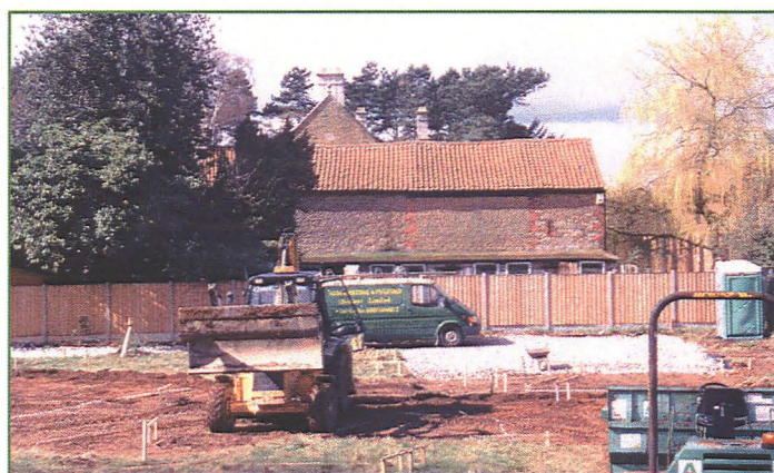
Plate 2 (left): General shot of the house footprint after excavation, looking SE, showing the barn to the rear of the Old House behind the boundary fence.
