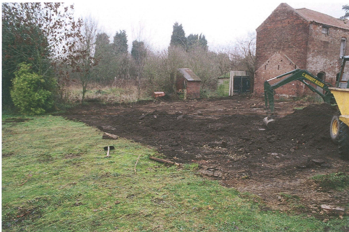
PI. 1 Topsoil stripping, ahead of footings excavation, photographed from the western site edge
