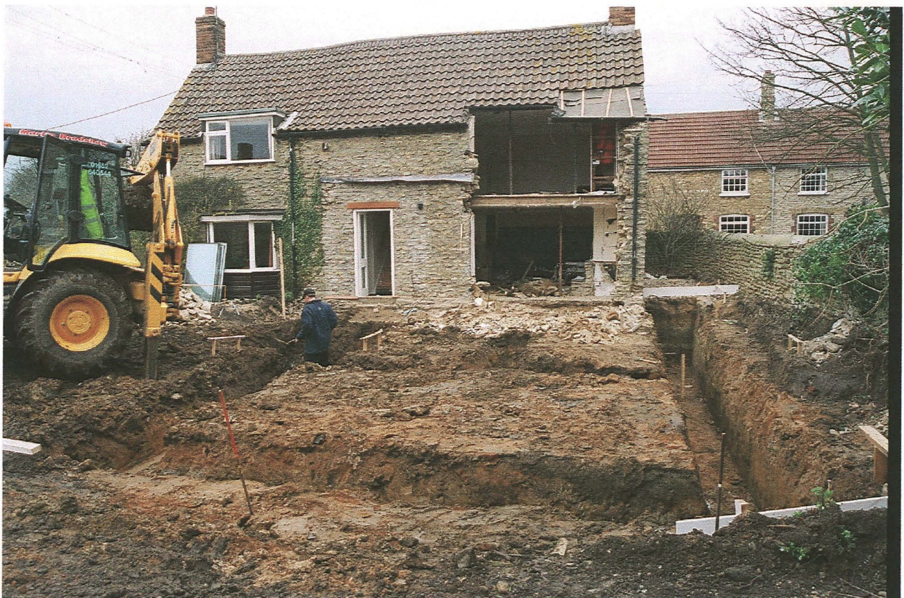
PI.4 View to the rear of the property, showing the demolished southern wall and partially completed excavation of the proposed foundations. Facing north.
