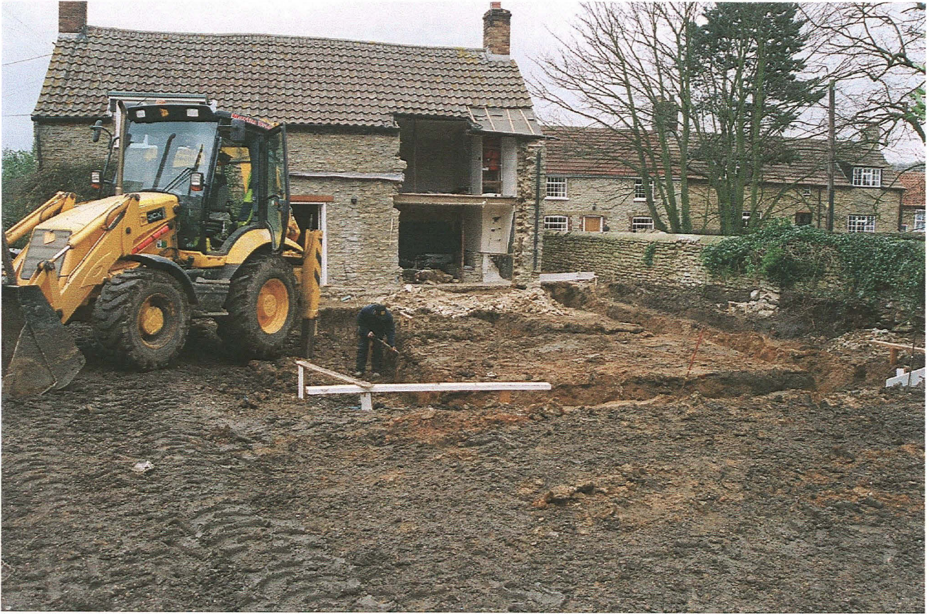
PI.3 View to the rear of the property, showing the demolished southern wall and partially completed excavation of the proposed foundations. Facing north east
