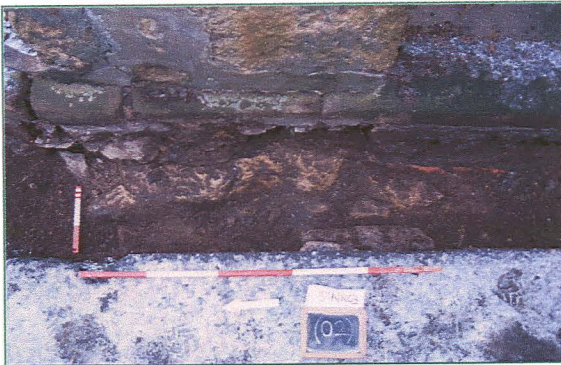
Pl.3. Stone foundation blocks, (002) at the base of the tower buttress, looking east.
