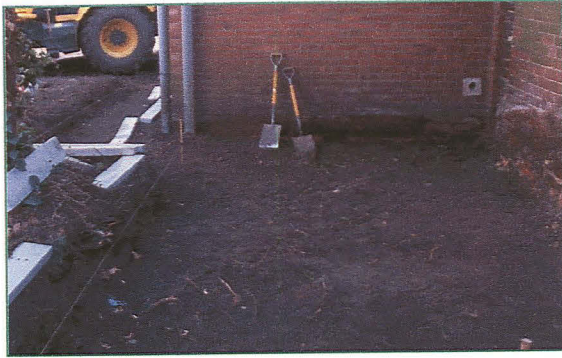
Pl. 1. Part of the completed groundworks in the south west corner of the church yard, looking east.
