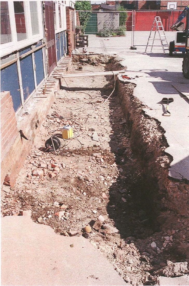
Pl. 1 (left) View of area backfilled with rubble prior to arrival on site, sondage excavated in bottom right of foundation trench, looking east.
