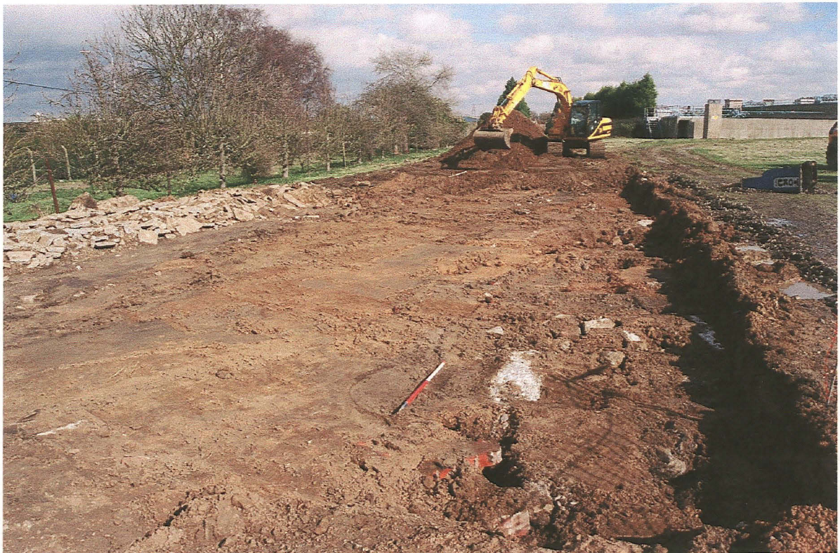
Pl. 8 Shot of area of development area to south of B119, looking east
