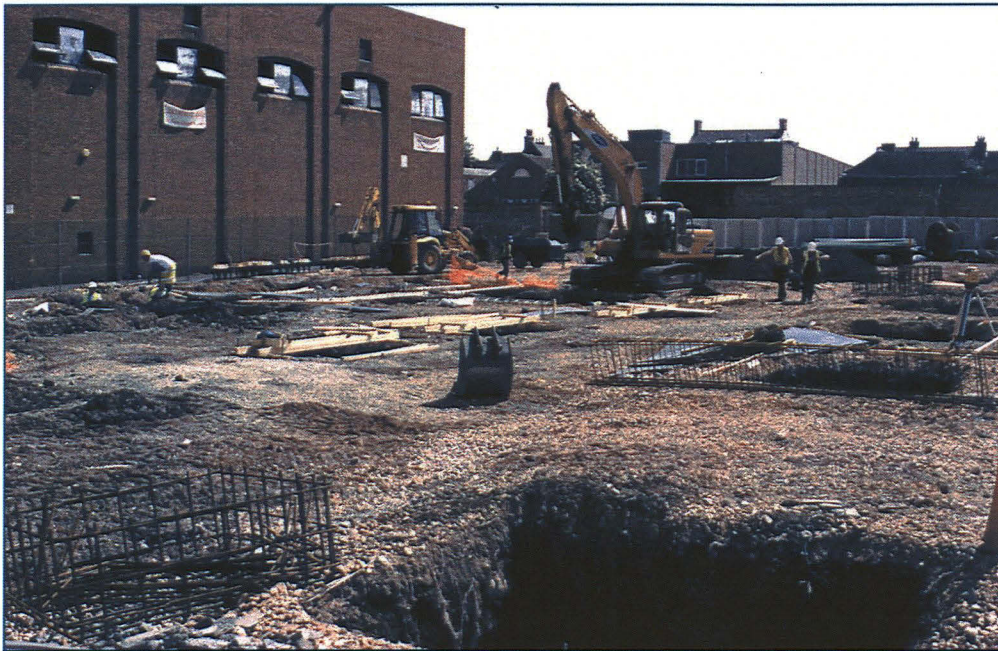
Pl. 1: General view of the development area, showing the foundation pits partially backfilled with concrete. Looking north-east
