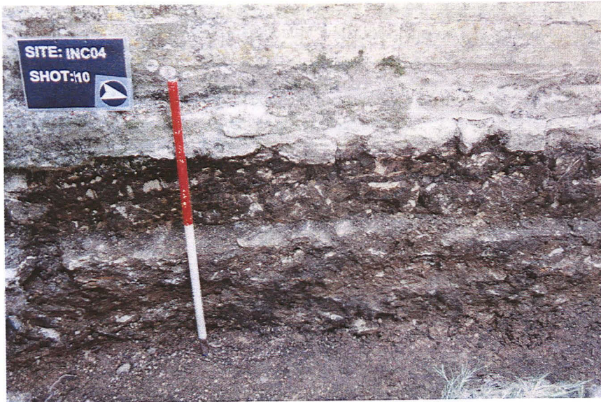
Plate 2 - Exposed foundations of the east wall of the north porch, looking west
