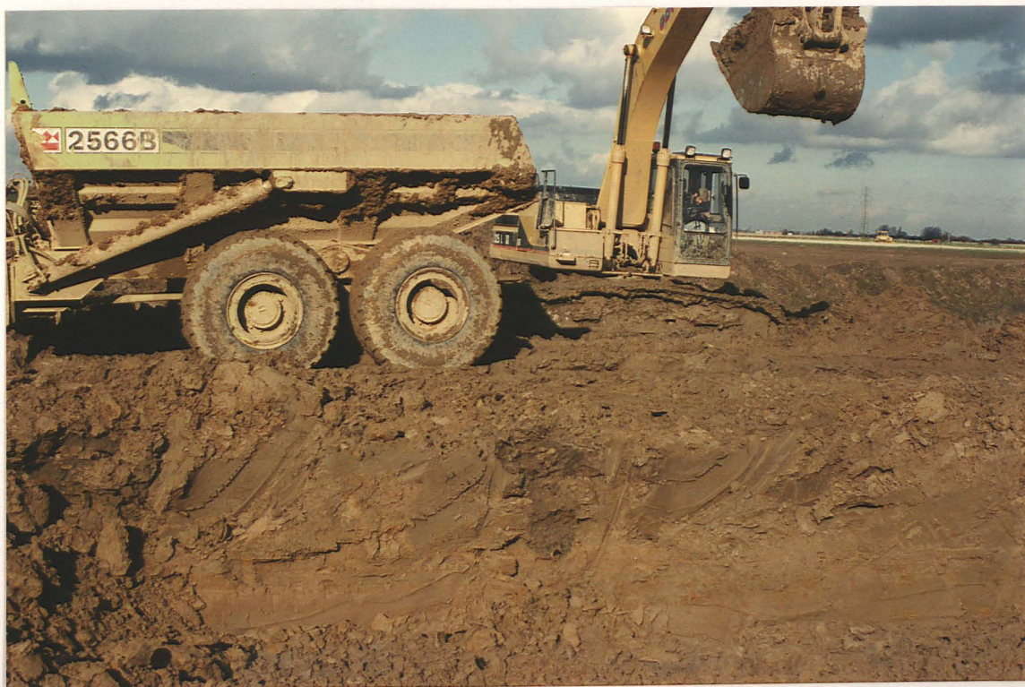
Pl. 34 The face of the borrowpit was too disturbed to permit identification of any features other than recent land drains.
