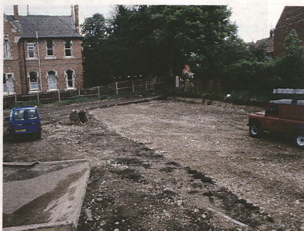
Plate 1. Northwest facing view across the site prior to the commencement of piling within Block A.
