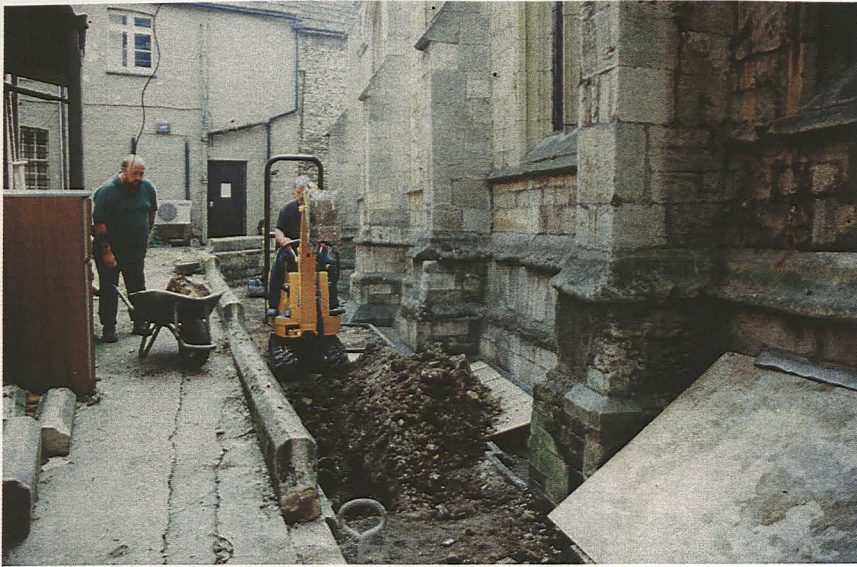
Plate 1 - General view of the drainage trench on the north side of the church, looking west
