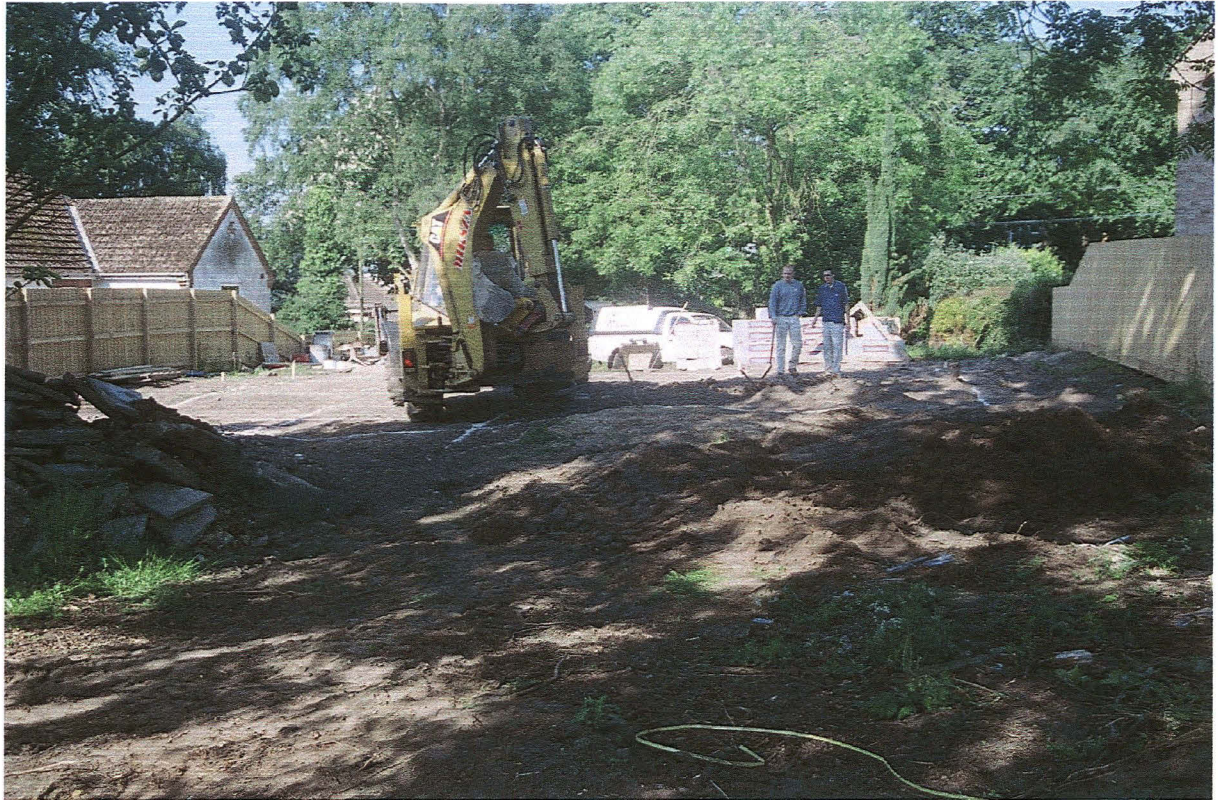
Pl. 1. The development site, after clearance of trees and partial topsoil stripping (looking west towards Church Lane from the eastern boundary).
