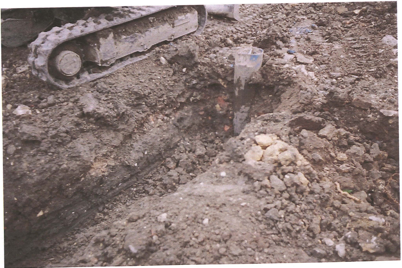
Pl. 10 A typical disturbed trench section
