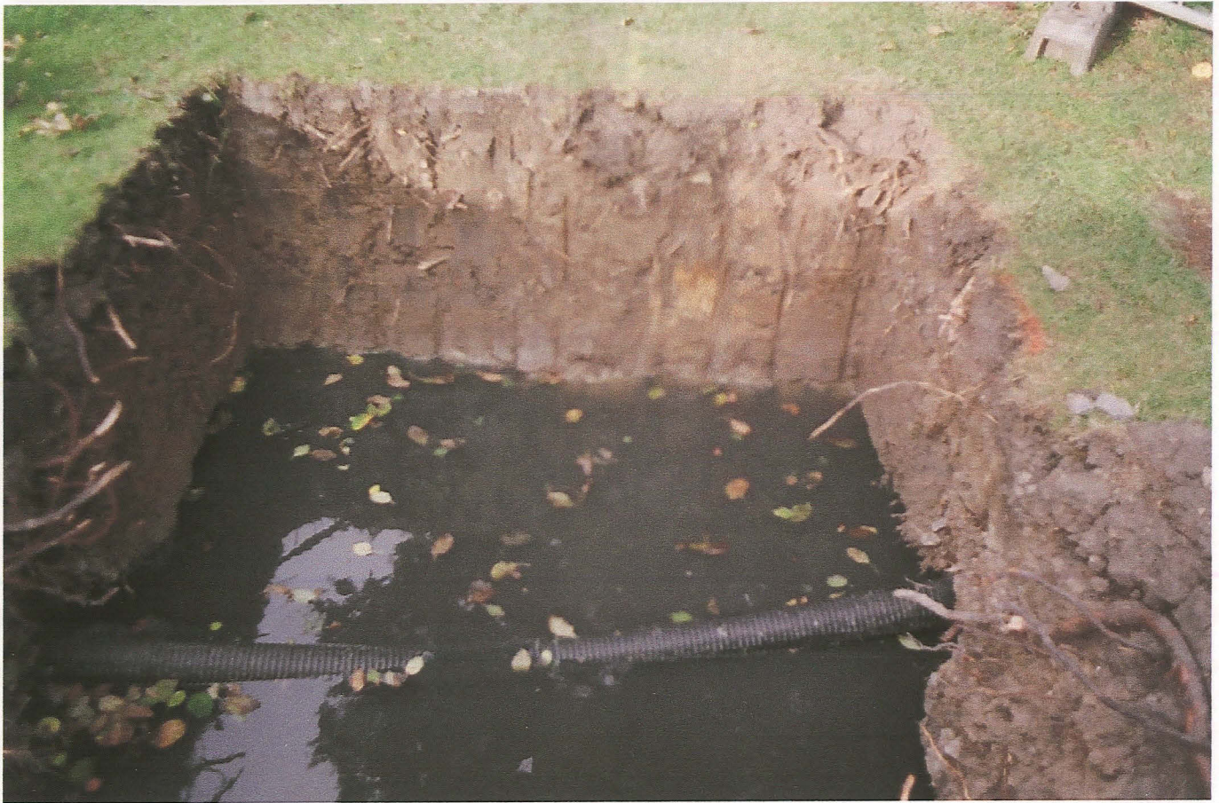
Pl. 3 Manhole 7 showing flooding from damaged land drains
