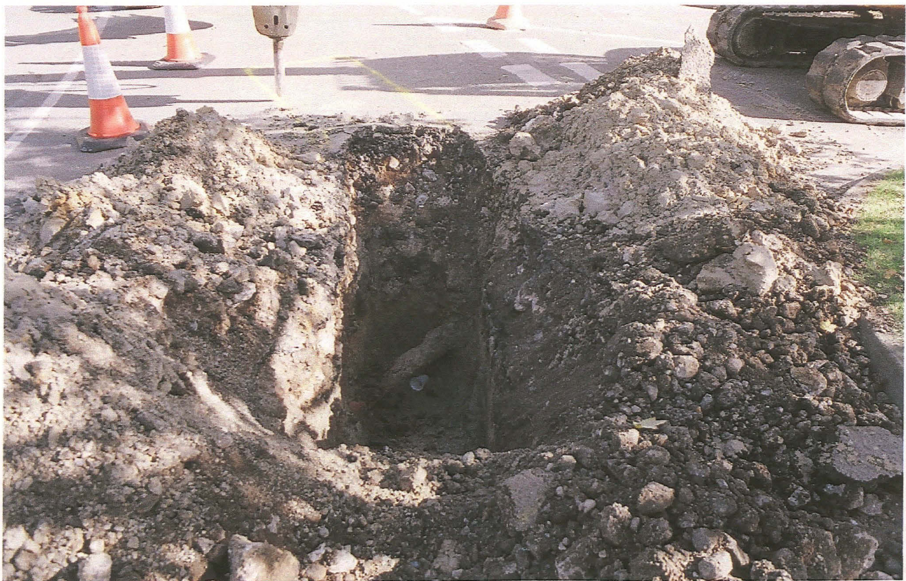
Fig 6. General view showing the deep nature of tarmac and road make-up along main street
