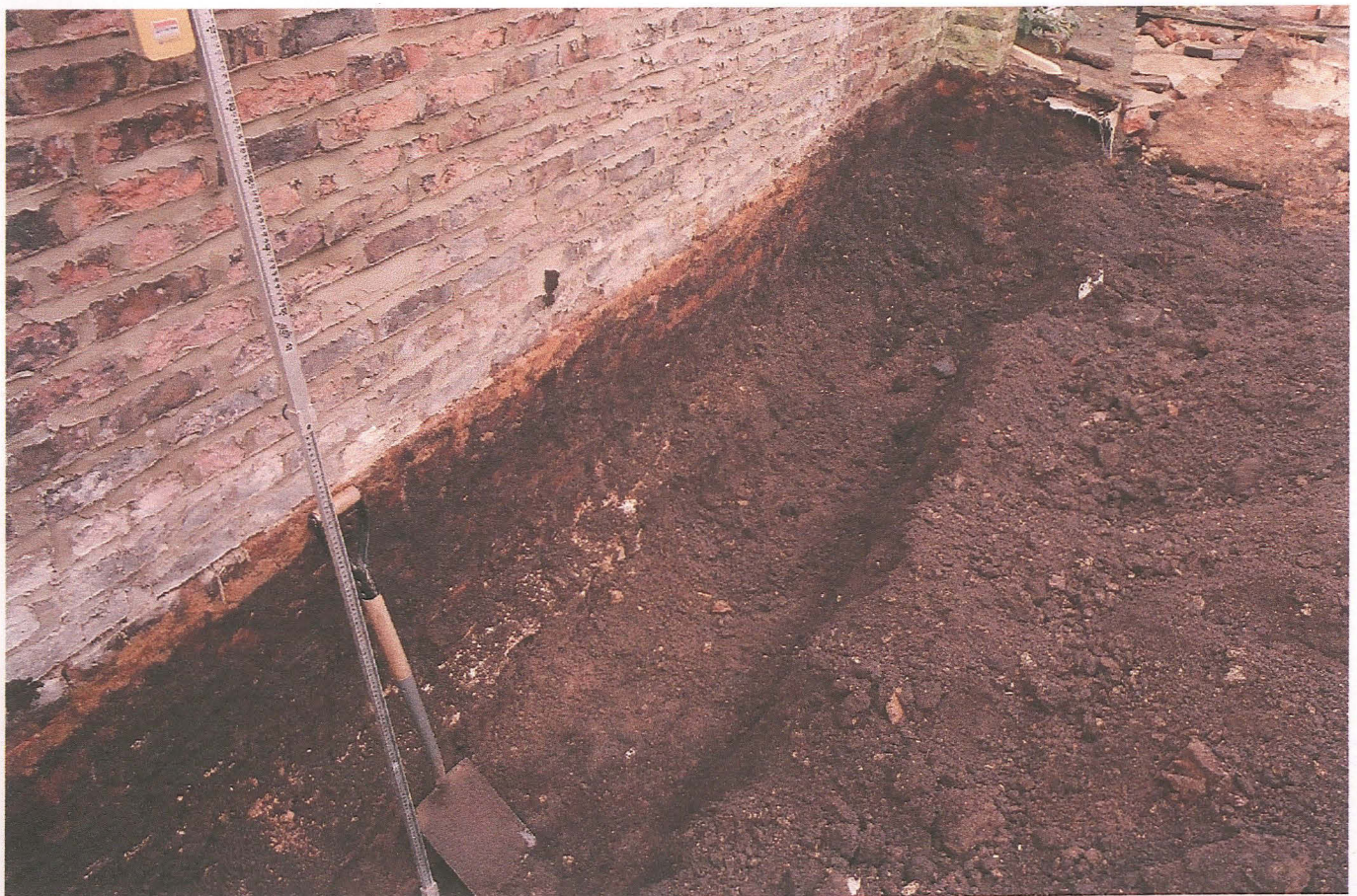
Fig. 6 Foundation trench showing final formation depth and stone foundations of boundary wall.
