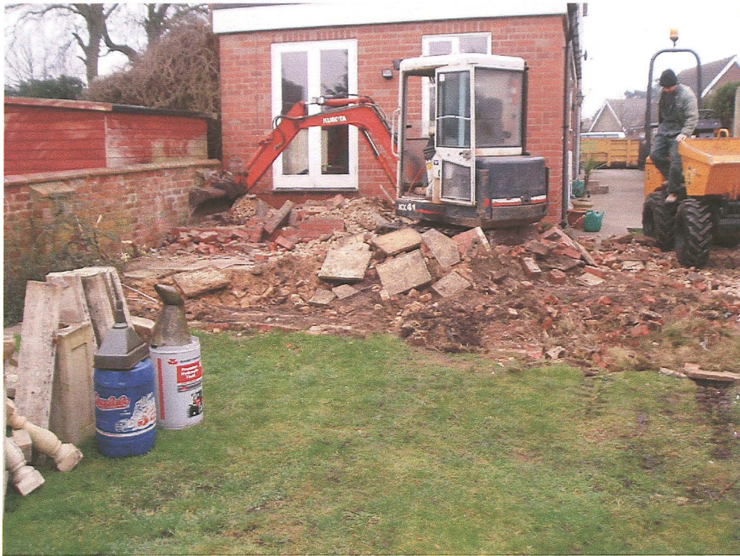
PI. 1 View of the rear of 60 Boston Road Horncastle during the removal of the patio, looking east.
