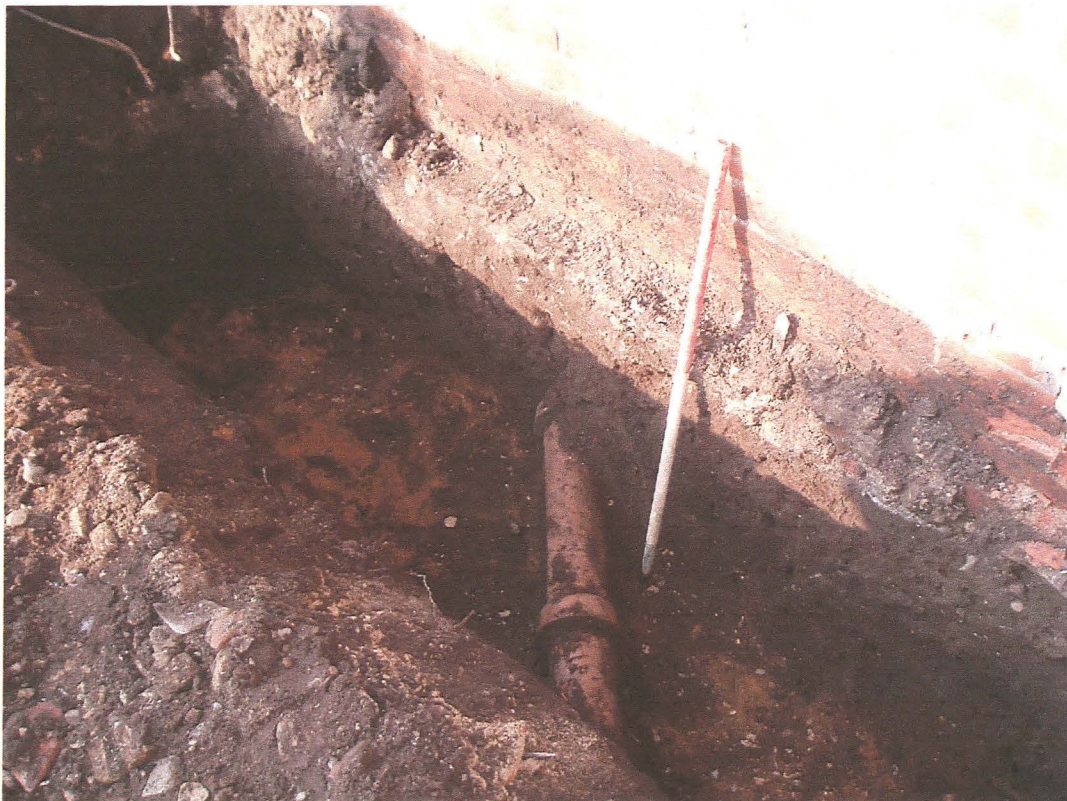
PI. 2 View of northern footing excavated to the natural sandy gravel (8), showing foundation of party wall, looking north (scale 1m).
