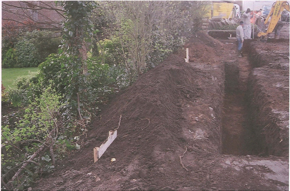
PI. 3 The depth of topsoil and subsoil increased towards the northern end of the foundation trenches. The lawn to the east is considerably lower than the development site, indicating probable artificial changes to the natural slope. Looking south along the eastern foundation trench.
