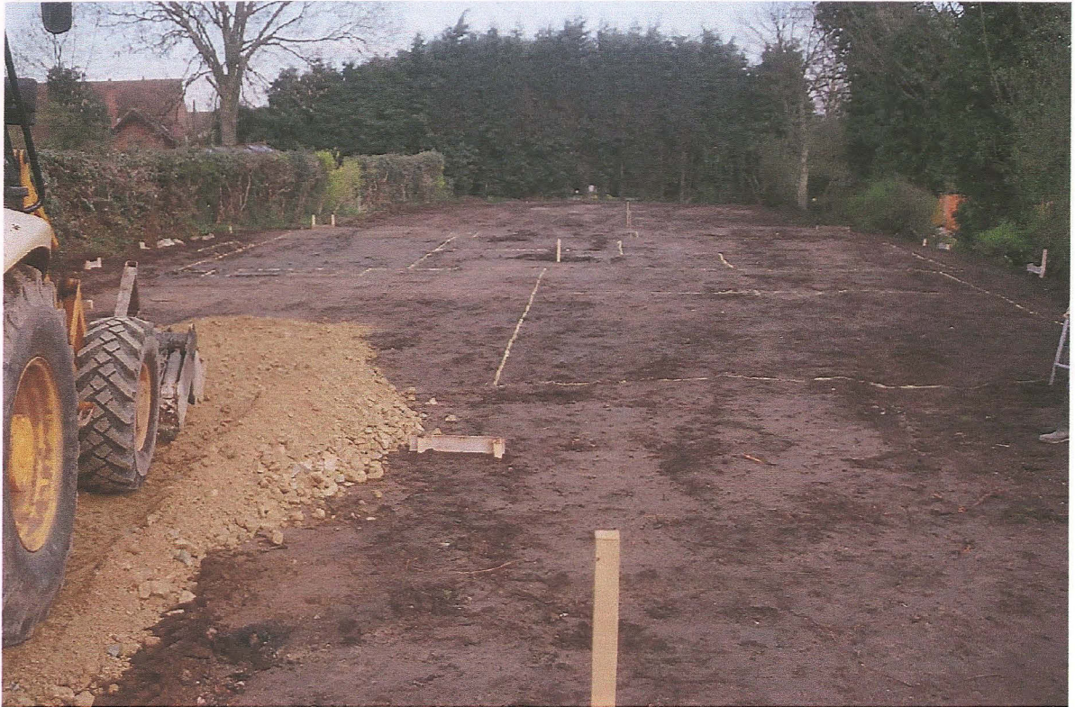
PI. 1 View of the development site after partial removal of topsoil, looking north.
