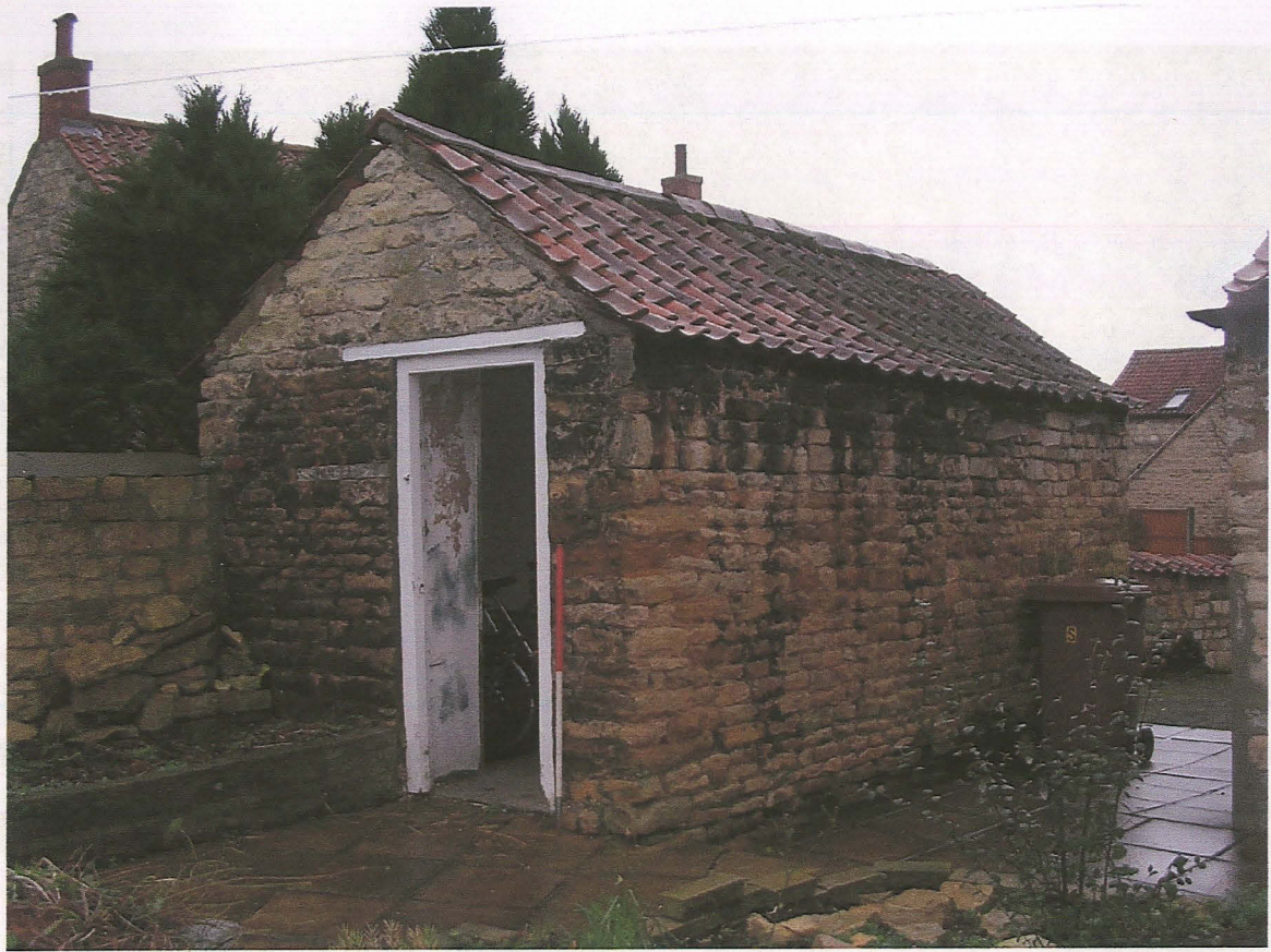
Pl. 9 The outbuilding, inserted door and rebuilt gable in east elevation, looking south west. Scale 1m
