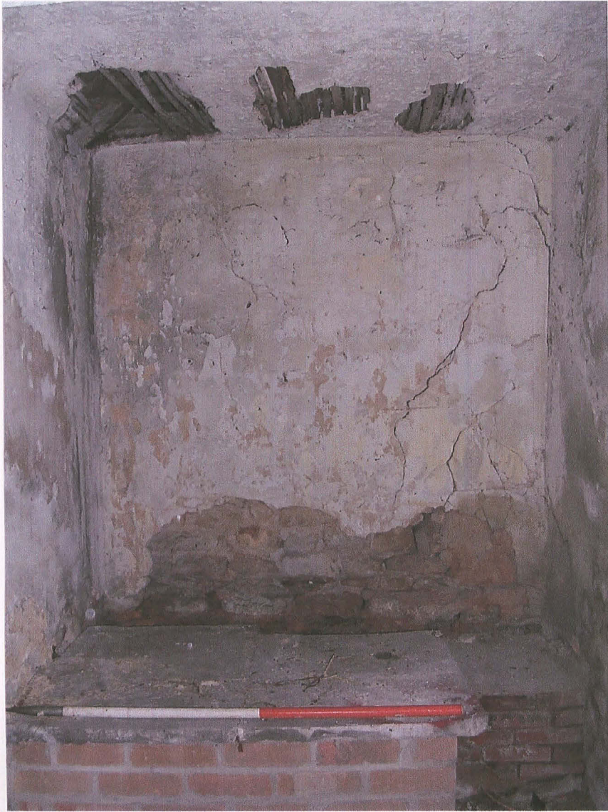
Pl. 13 Interior of west half of outbuilding, looking east. Plinth for oil tank in front of brick bench. Scale 1m
