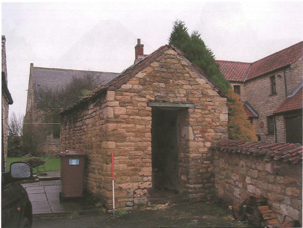
Pl. 8 The outbuilding north and west elevations, looking east. Note raised gable and rebuilding above door lintel. Scale 1m
