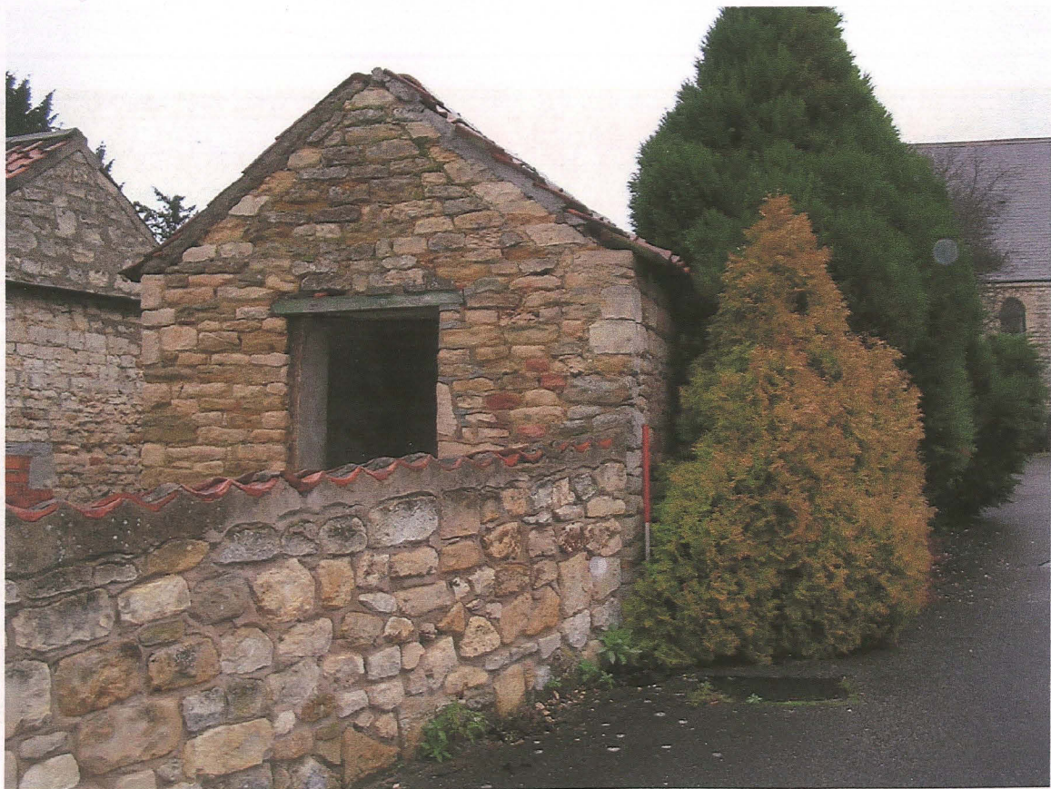
Pl. 10 Outbuilding in relation to later boundary wall which butts southwest corner of building. Looking east. Scale 1m
