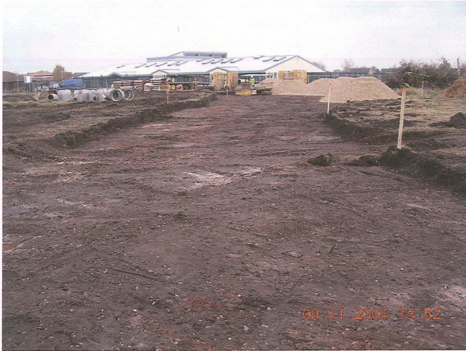
Pl. 3 Topsoil stripping for the access road revealed no archaeological features (looking south-east towards the school).
