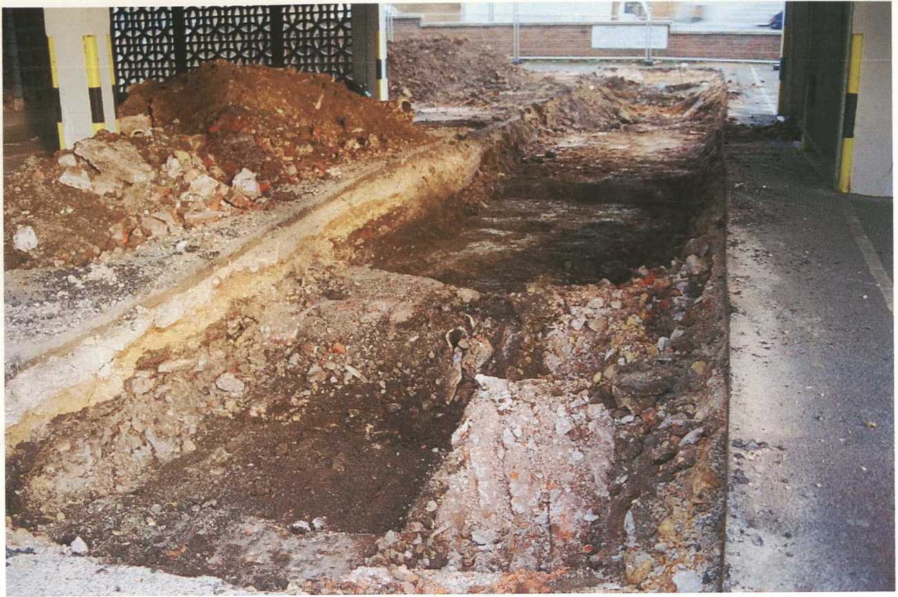
Pl. 1 General view of trench looking east, before cleaning, with concrete 107 in foreground. Note broken sewer pipe in centre which originally ran along the length of the trench.
