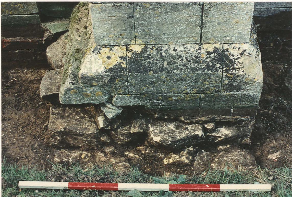
Pl. 44. Foundations beneath S aisle buttress marking position of earlier S transept (S side).
