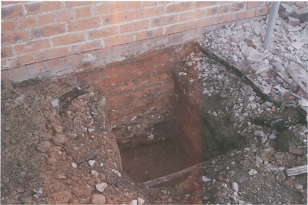
PI. 15 Trench G exposed the foundations of the adjacent surviving building (looking east).
