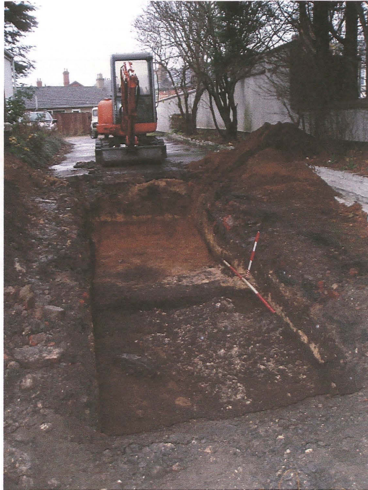
Pl. 5 General view of trench. Limestone rubble 110 cut by later features (113, 116, 118 and 120). Looking north-west. Horizontal scale 2m, vertical scale 0.50m.
