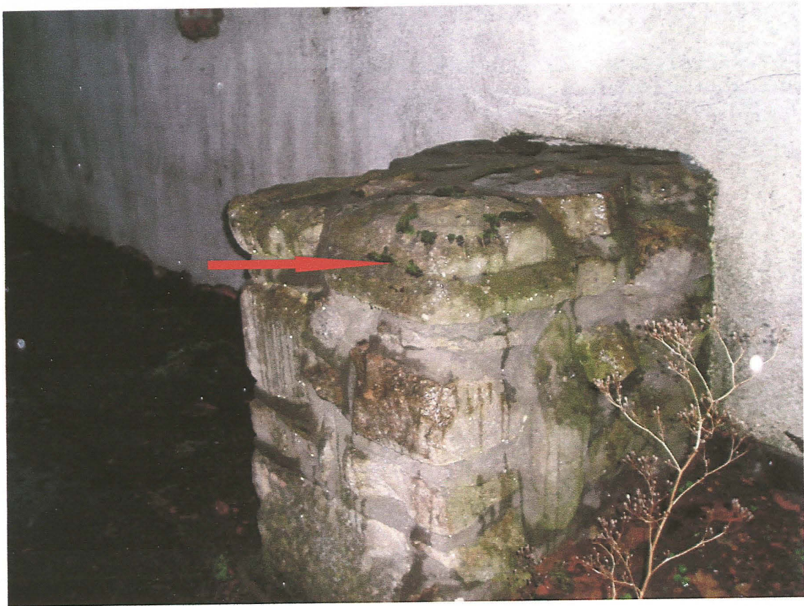
Pl. 15 Detail of pier 2 showing possible column capital on top of the pier (upside down). Looking northwest.
