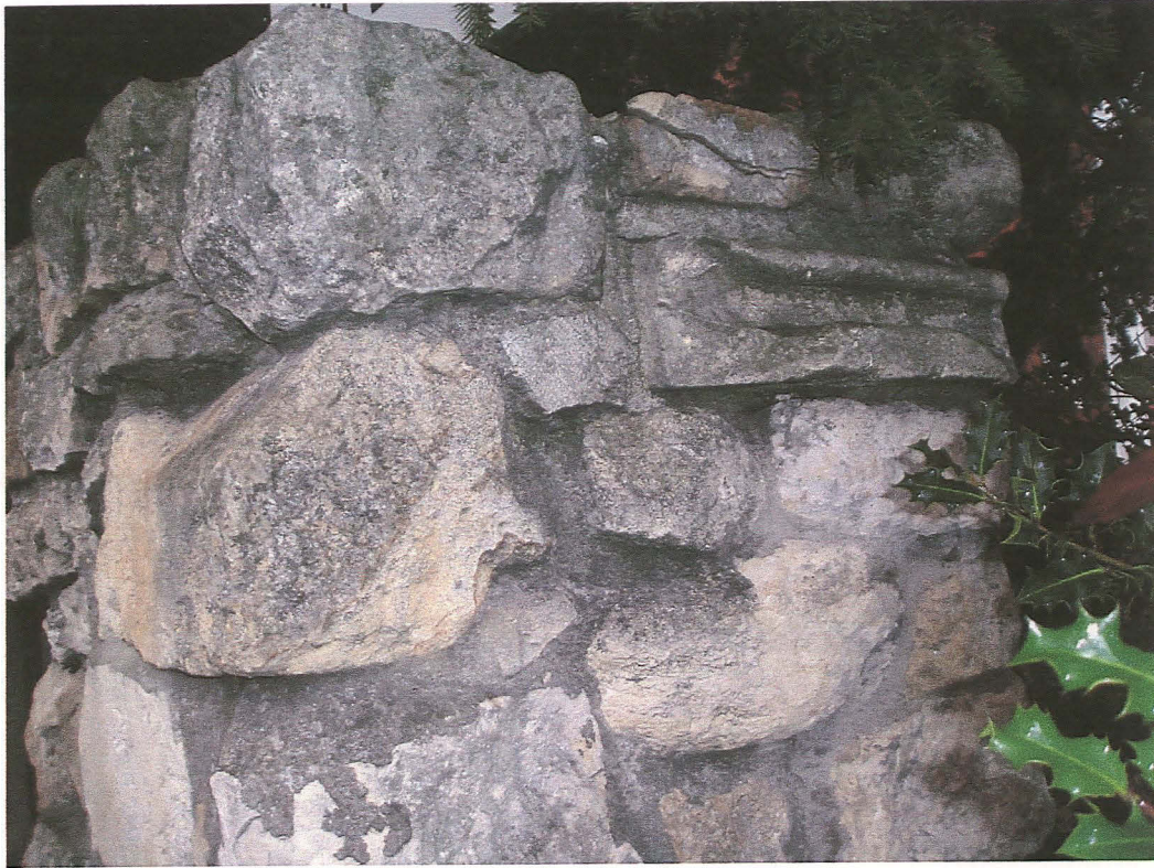
Pl. 13 Detail of pier 1 showing architectural fragment close to the top of the east face (right hand side).
