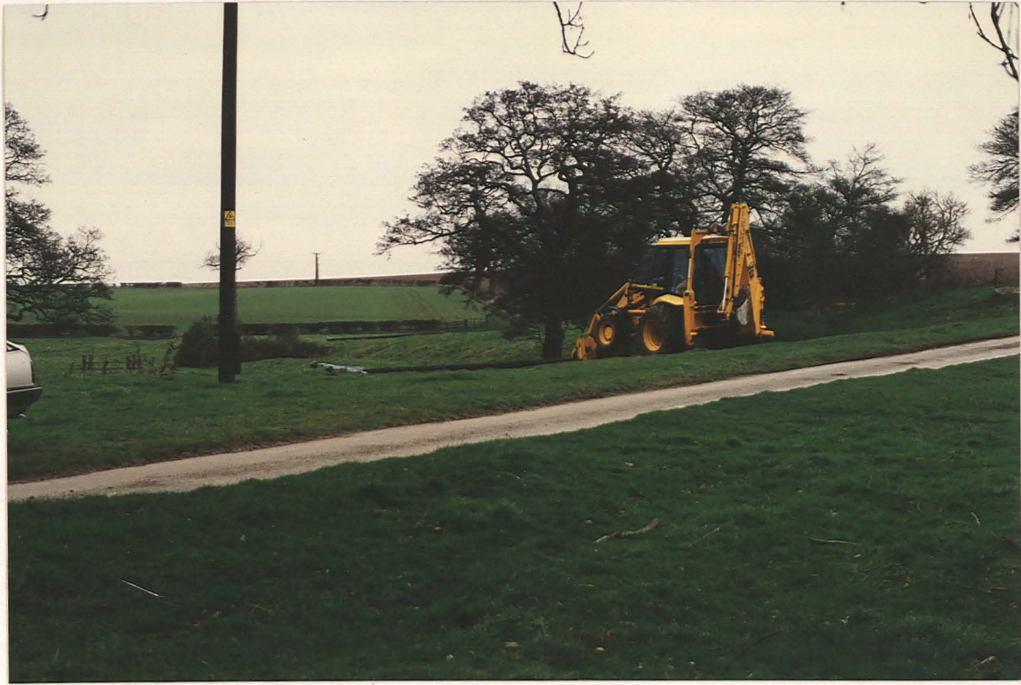
Pl. 2 Driby, general view of monitored area with existing poles (looking north from the road)
