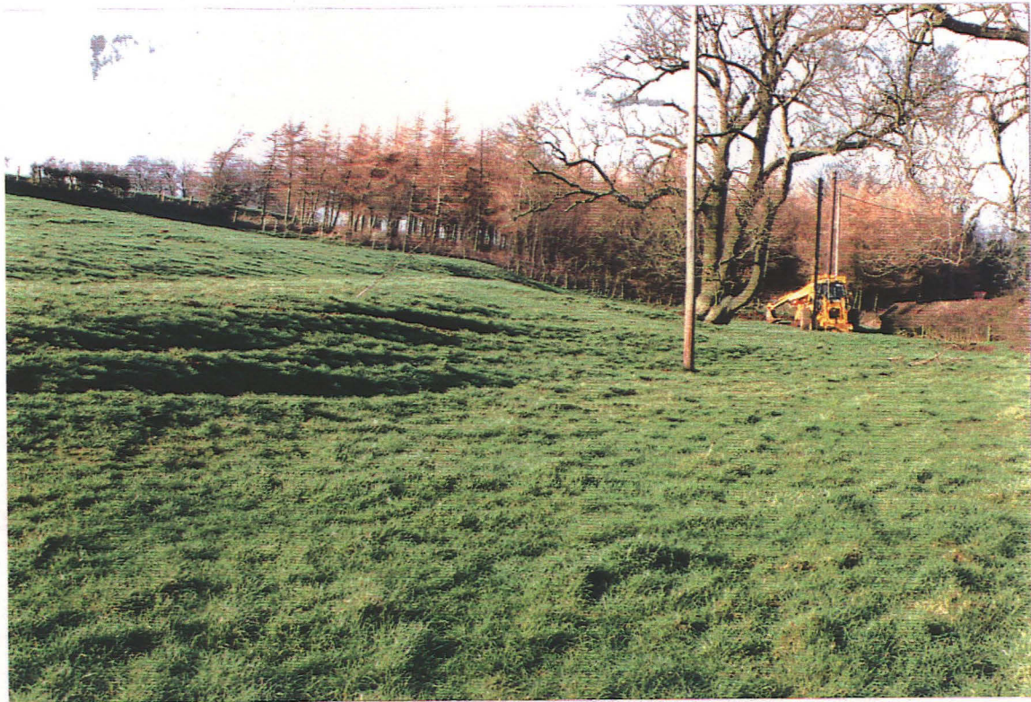
Pl. 43 Natural valley to north of Brinkhill Road; the depression in the foreground was very wet. The excavator is beside Holes 35-37 (looking west)
