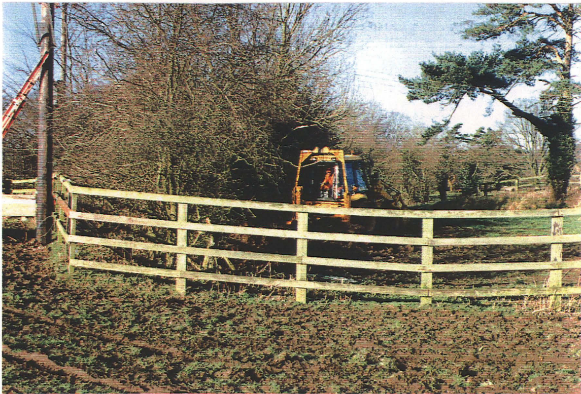
Pl. 41 Location of Hole 33 (ladder against new pole) with excavator cutting Hole 34 (looking west)
