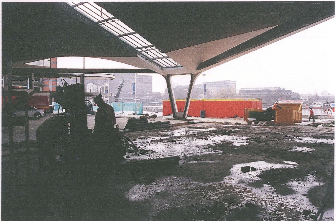
Pl. 2 Looking north at the interior of the development with the Brayford Pool to the south
