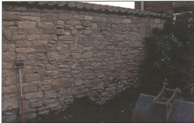
Pl. 4: East end of the boundary wall. The scar defining a former wall is visible to the immediate left of the scale. To the east, a repair in smaller stones is evident. Looking north-east.
