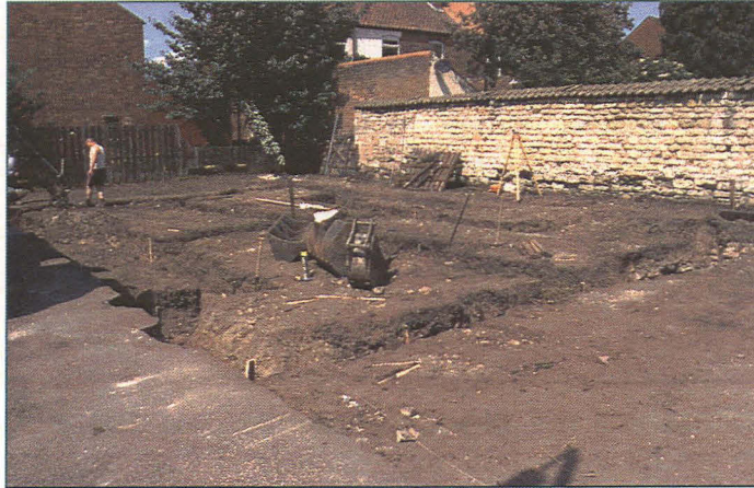
Pl. 1: General view of the development area after excavation of the footings. Looking north-west
