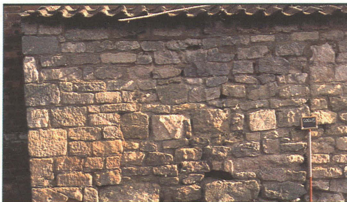
Pl. 3: West end of the boundary wall, looking north. The scar indicating a possible wall running south is visible above the scale.
