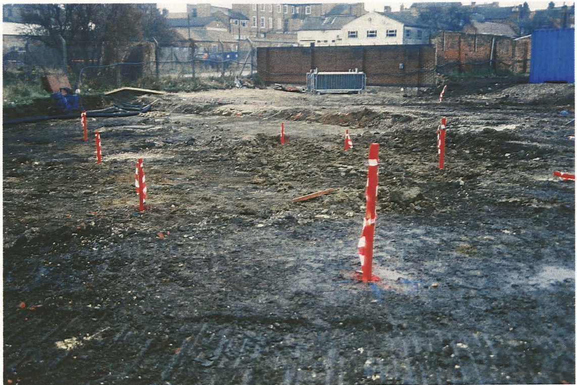
Plate 3 General view of exposed concrete culvert, and line of new culvert trench, looking north-east
