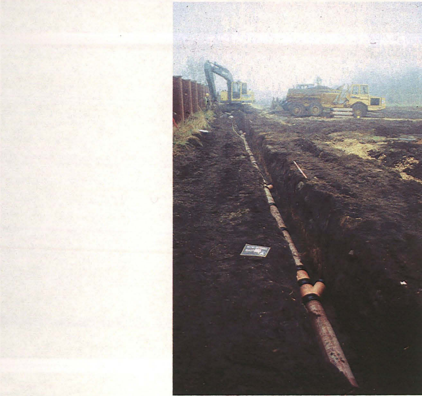
Plate 23 North facing view drain run MH7 to MH8 showing working conditions during watching brief.
