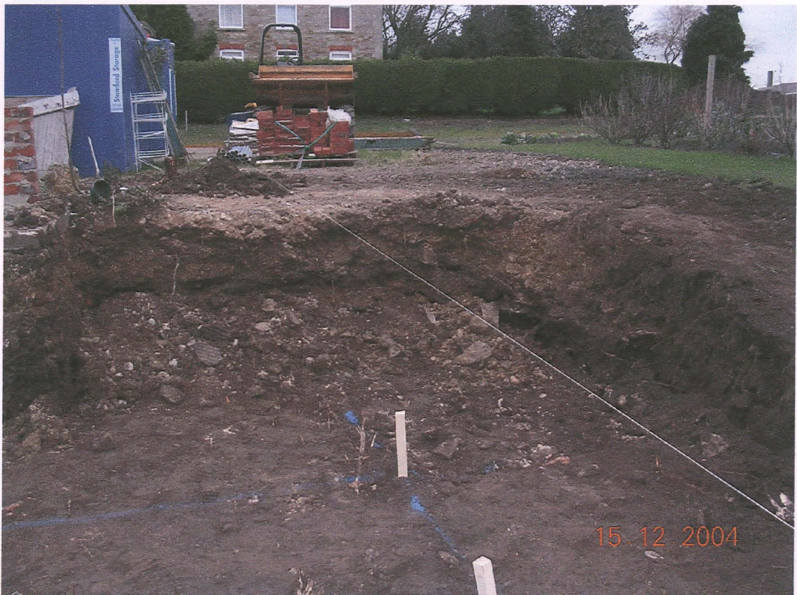
PI. 4 North-eastern corner of the area stripped for the retaining wall (looking north). Rubble from the soakaway 9 is visible. The sloping ground to the north appears to have been lowered when the garage was built.
