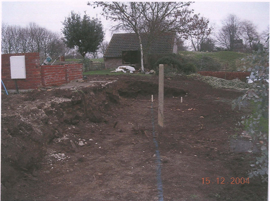
PI. 3 Area stripped for the retaining wall (looking east towards the castle site).
