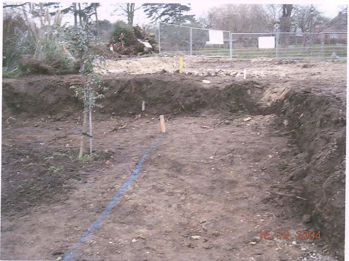
PI. 2 Area stripped of topsoil for the new retaining wall (looking west towards Bourne Road).
