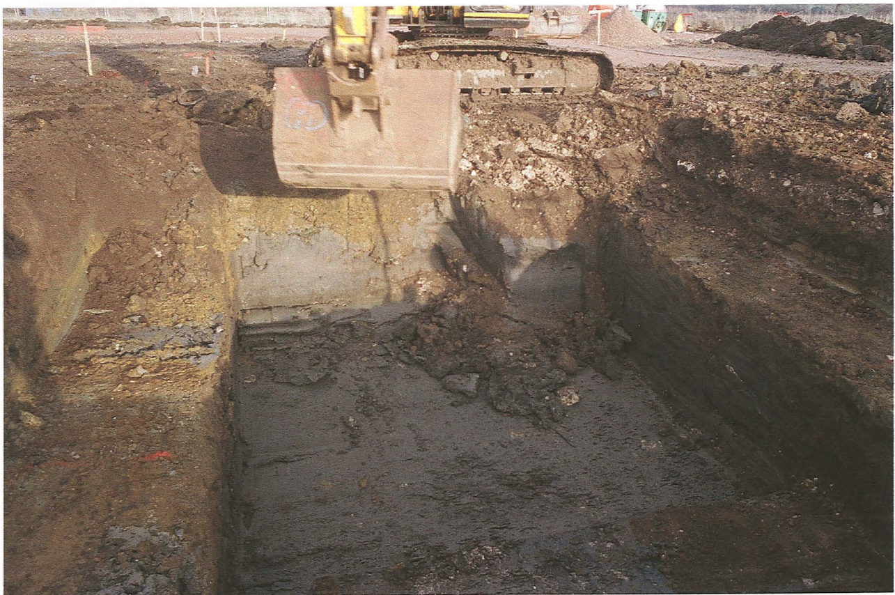
Pl. 6 Excavation of a large pit for main storage tank behind the poultry farm on Back Lane
