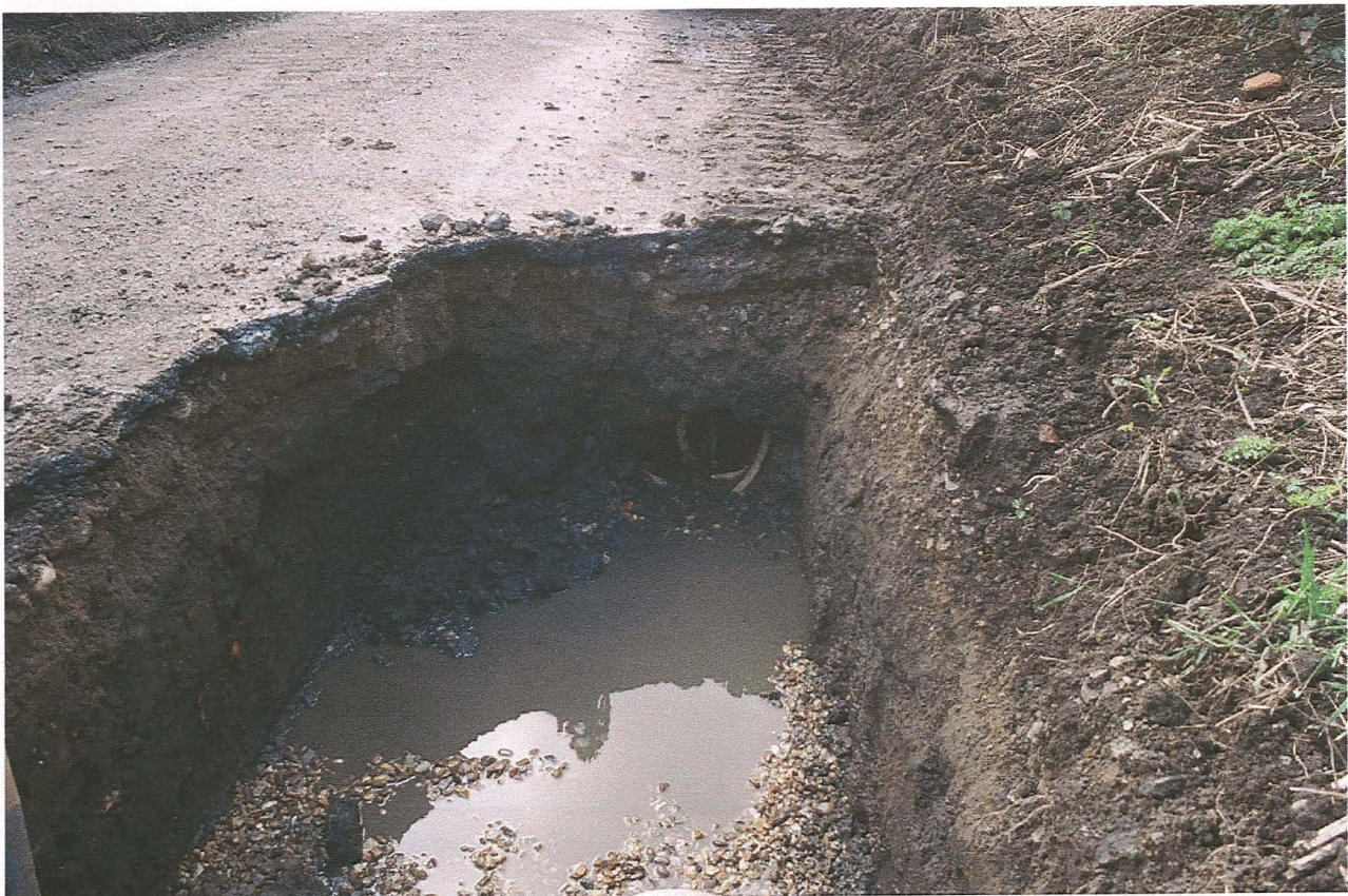
Pl. 14 Fractured drainage pipe in Back Lane adjacent to The Row
