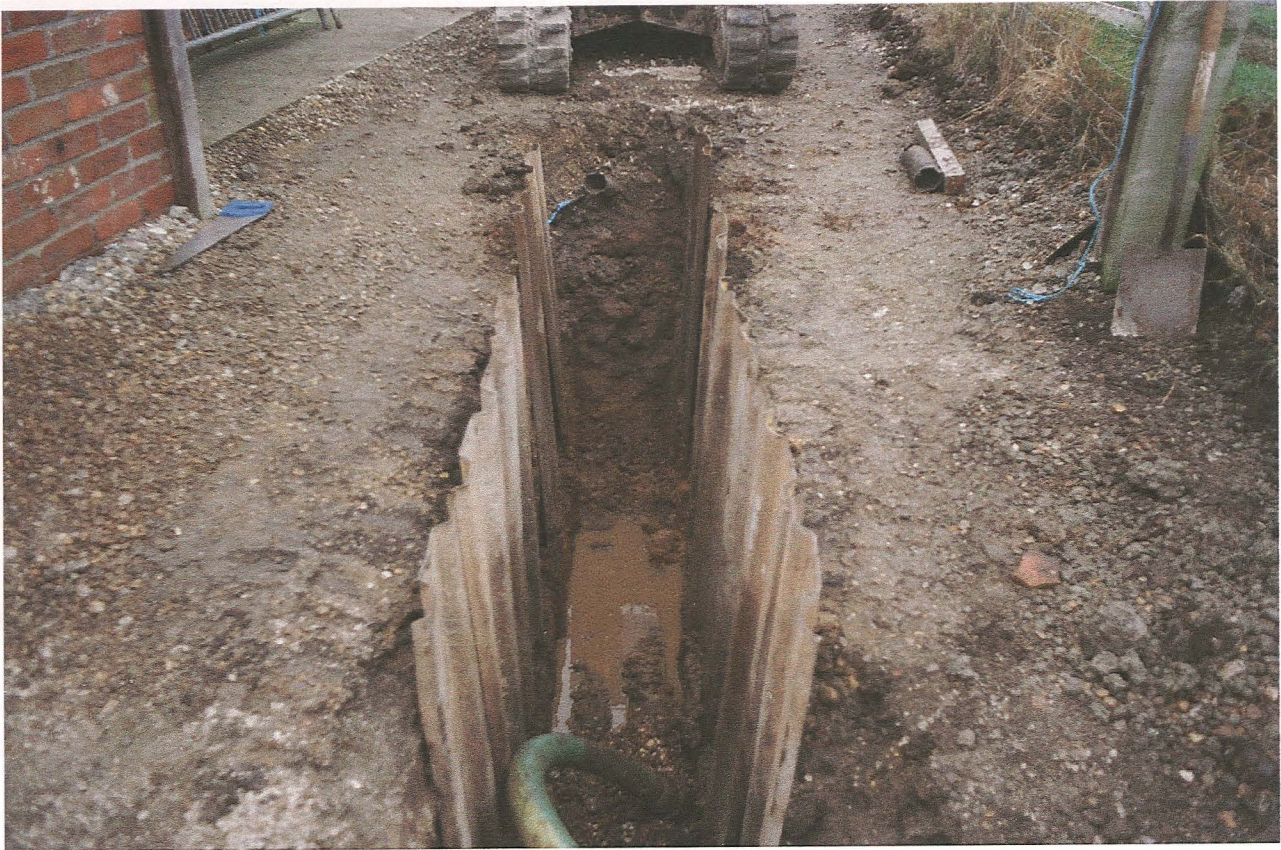
Pl. 13 Open cut trench running south along the driveway of Hope Cottage off Dukes Head Lane
