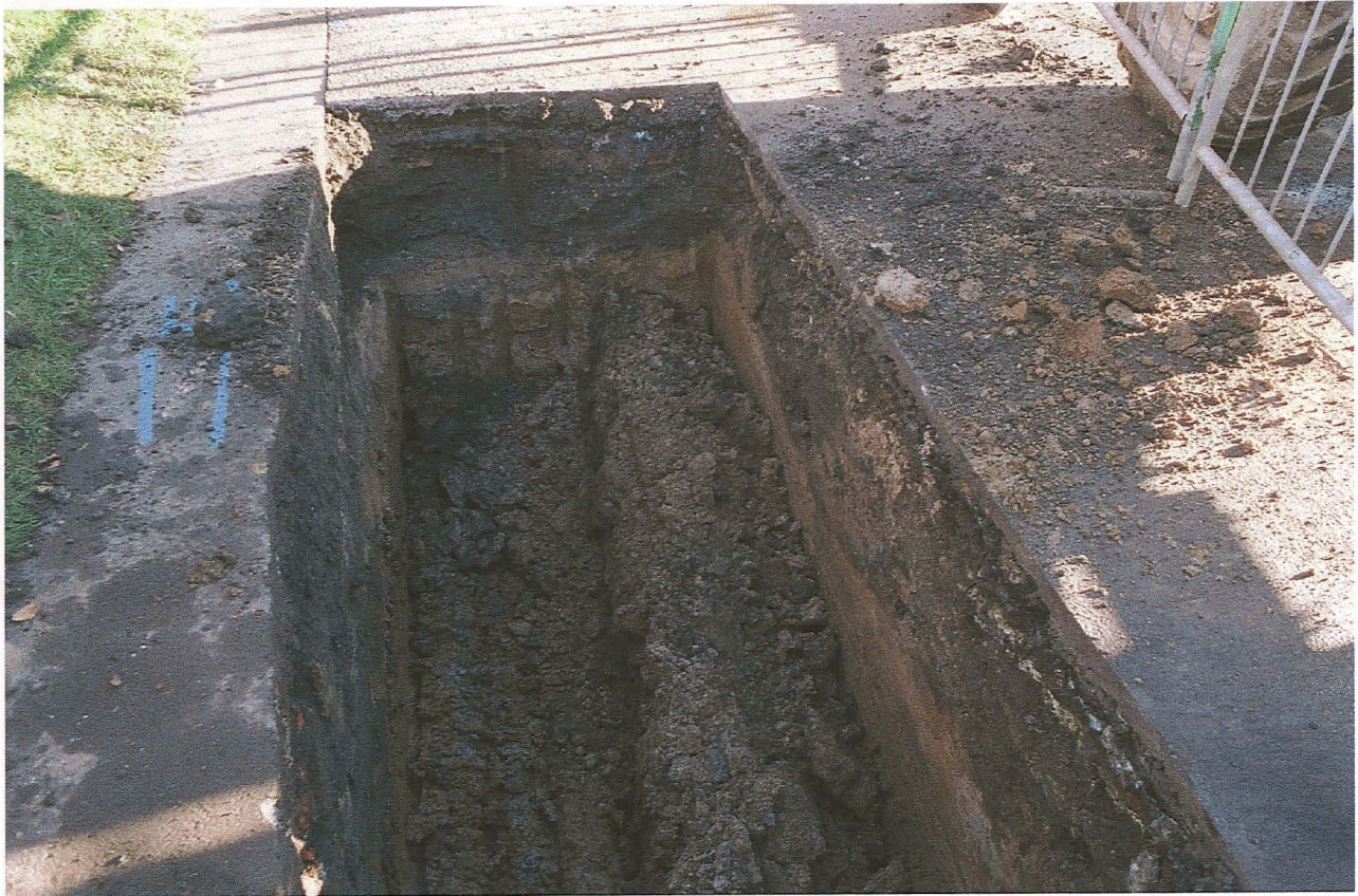
Pl. 11 Looking south along Hagnaby Road showing road build-up overlying sandy silts that seal natural dark boulder clay
