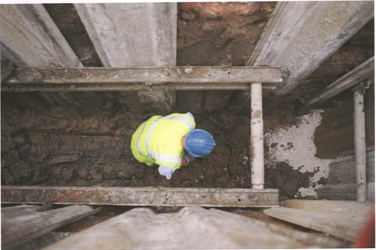
PI. 19 Photograph demonstrating the depth of the open cut trench along Moat Lane
