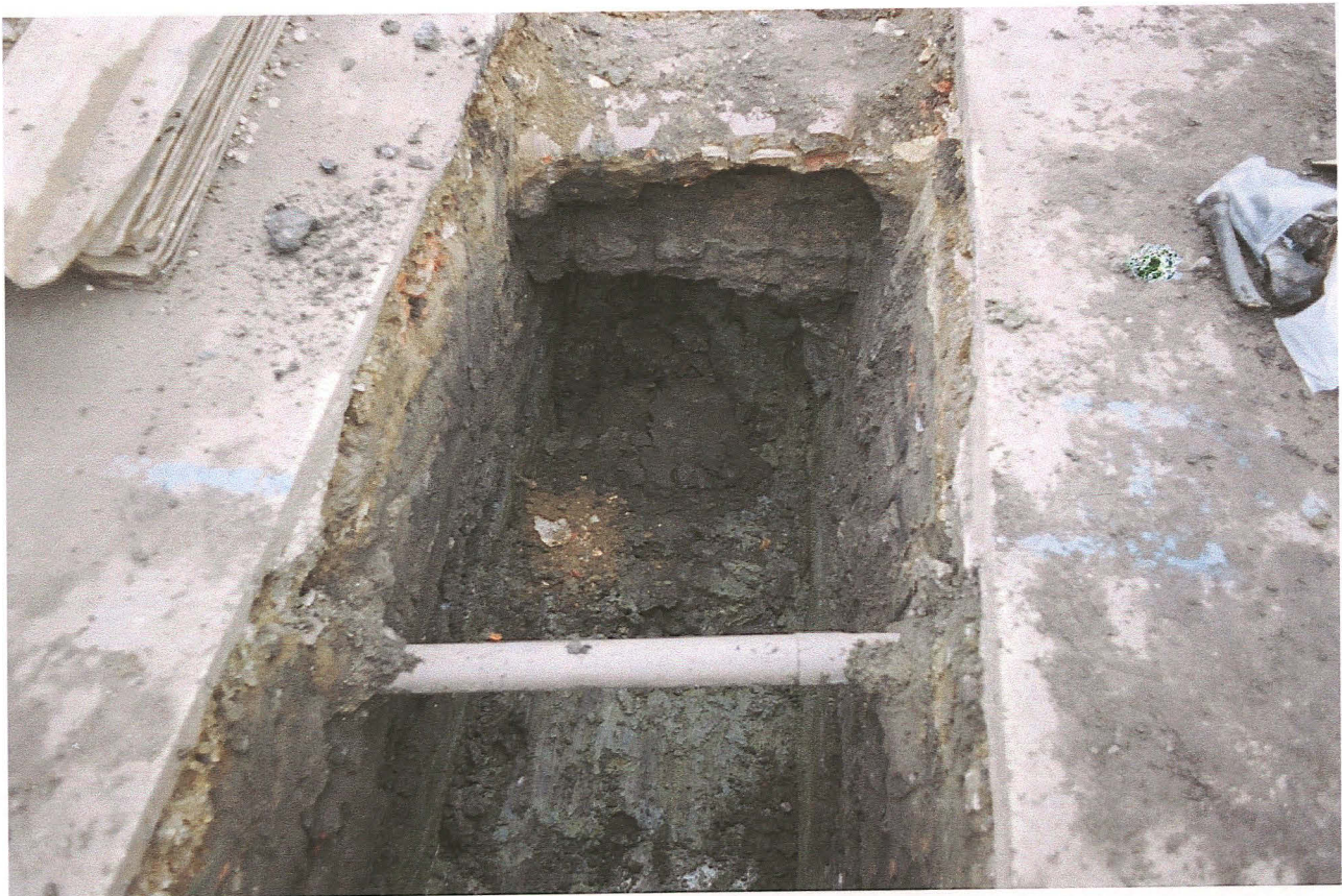
Pl. 18 General view showing stratigraphy and services at the junction between West Keal Road and Main Street
