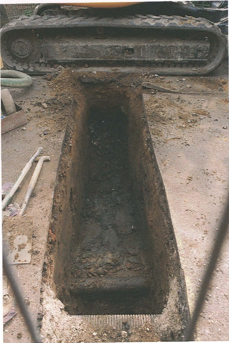
Pl. 15 Looking west along open cut trench on Back Lane adjacent to Greenbank
