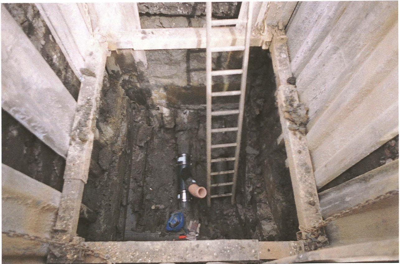
Pl. 22 Photograph demonstrating the depth of manhole C2 at the northern end of Moat Lane
