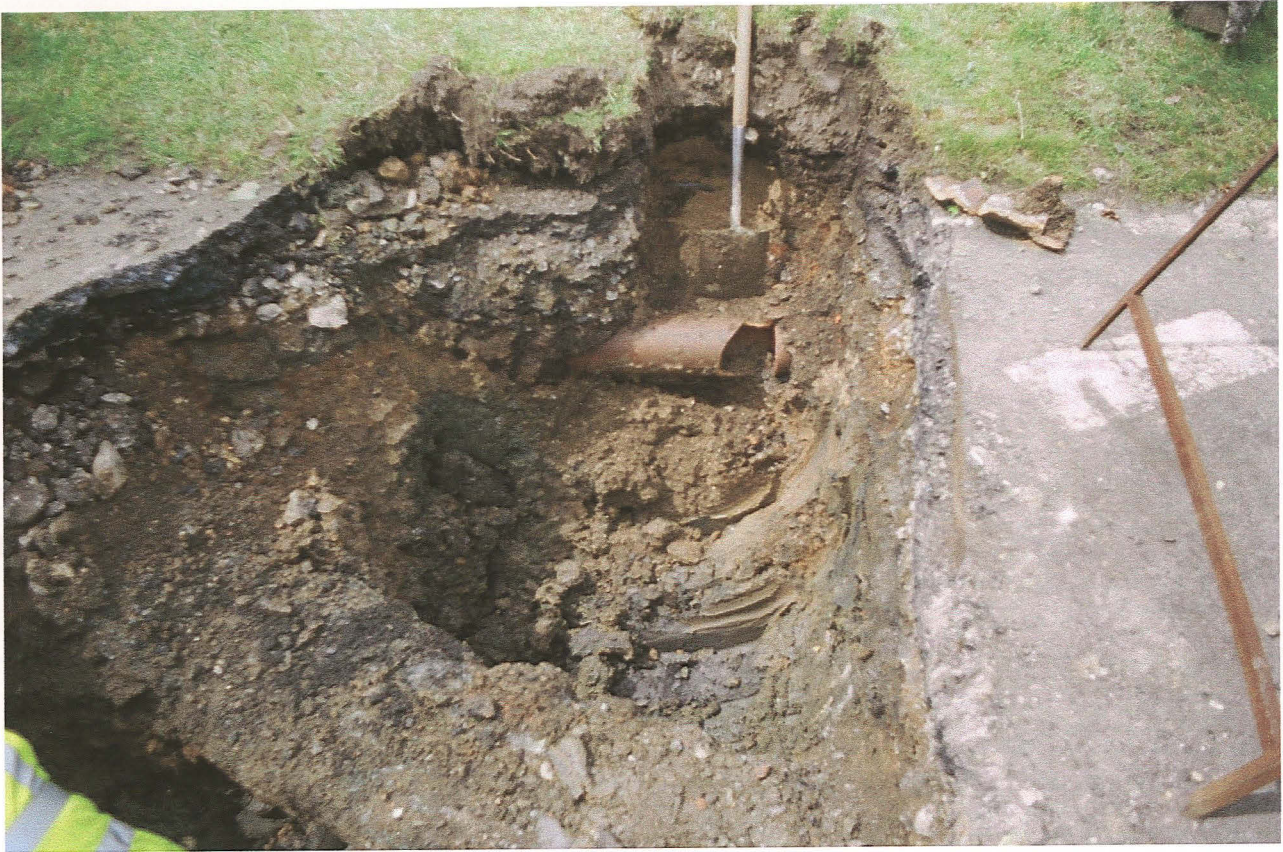
Pl. 21 Photograph showing disturbance and services at the junction between Spilsby Hill and Church Lane
