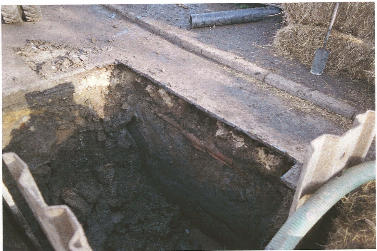
Pl. 8 Manhole A4 on Hagnaby Road showing rough stone deposit and land drain in eastern baulk
