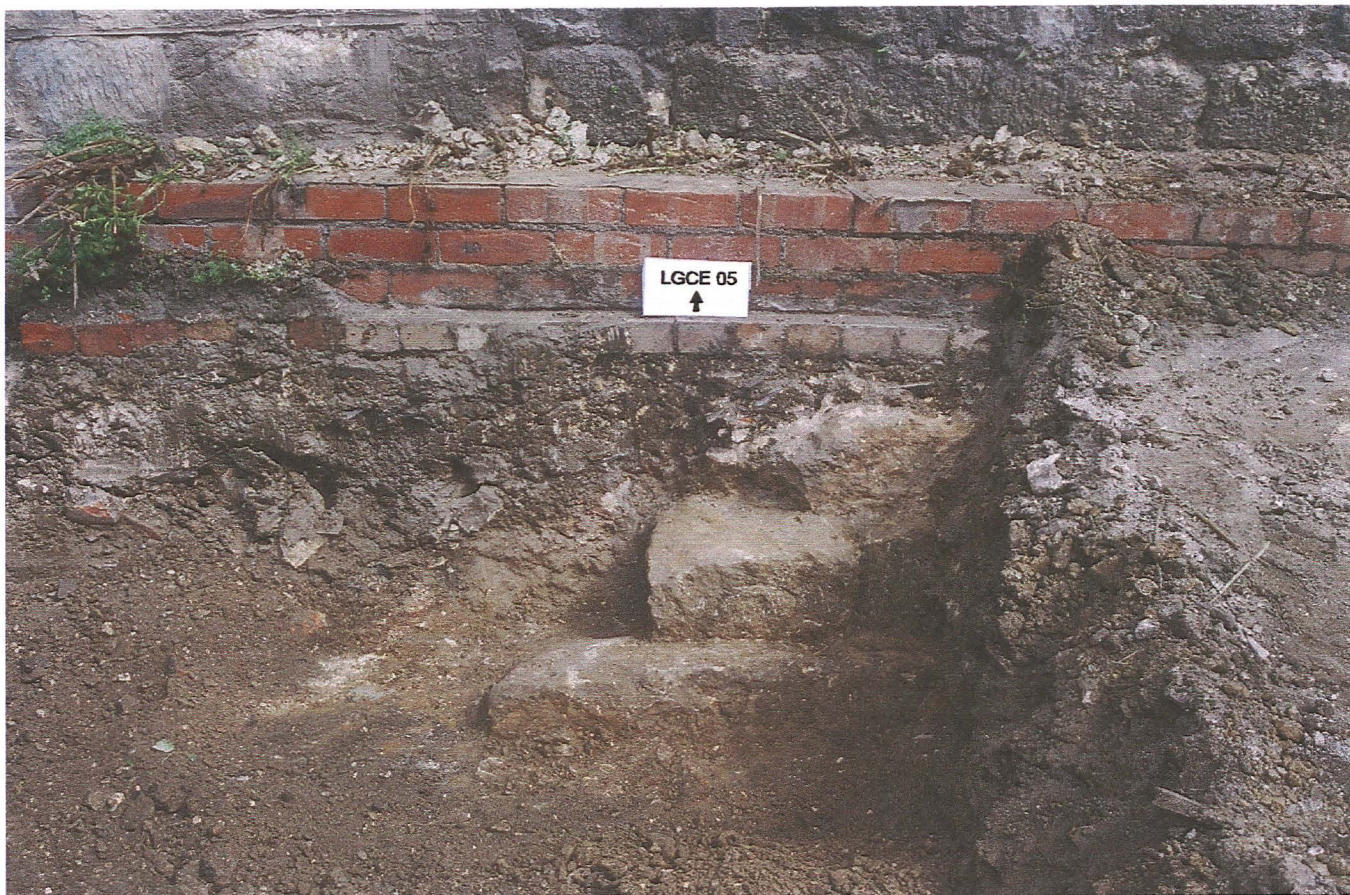
Pl. 18 Extension to Trench 1 showing the junction of the intact Close Wall foundations (right) with the robbed area to area to the left and modern brick underpinning above
