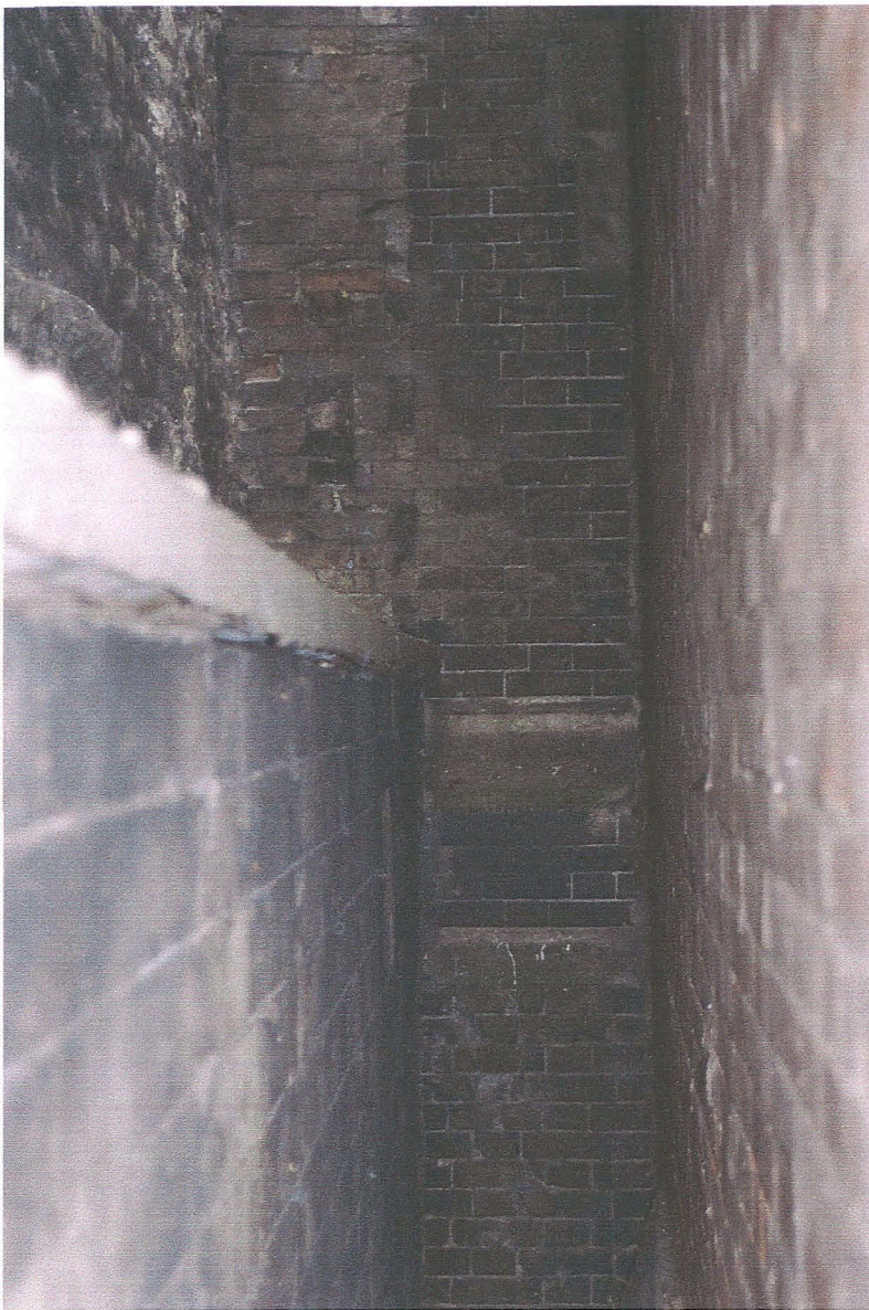
Pl. 20 The view between the north wall of the art college and the orangery wall showing the probable chimney for the fire room at the eastern end
