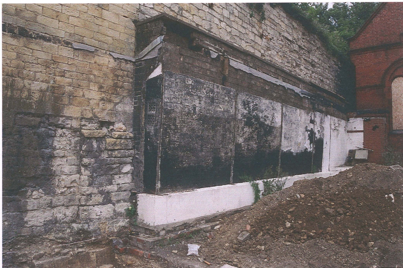
Pl. 19 Looking east towards the art college showing the close wall and surviving rear wall of the orangery
